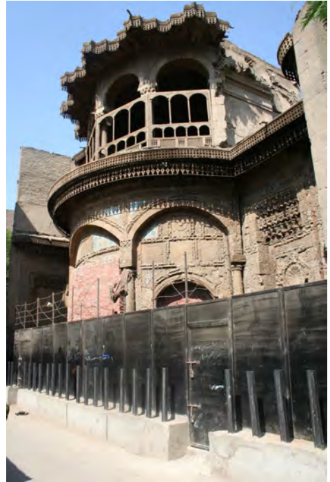
Figure 9.5 Sabil of Ruqayyah Dudu, Cairo, is a neglected sabil that was robbed of its metal grilles and other architectural fixtures; conservation professionals have put up a fence and barbed wire to protect it from further vandalism and theft. Image: Hossam Mahdy
