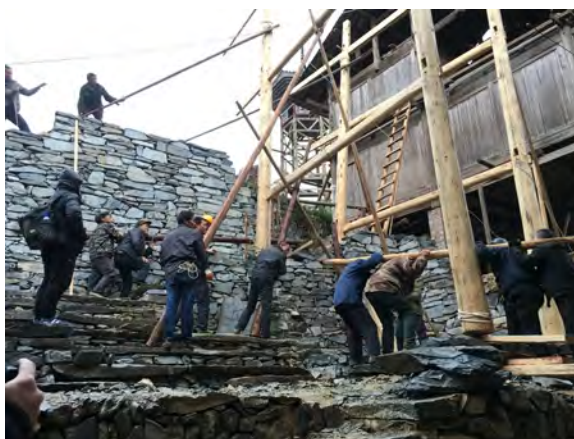
Figure 7.4 Construction of a traditional chuandou structure in Dali village by the villagers. Image: © Li Kuanghan
