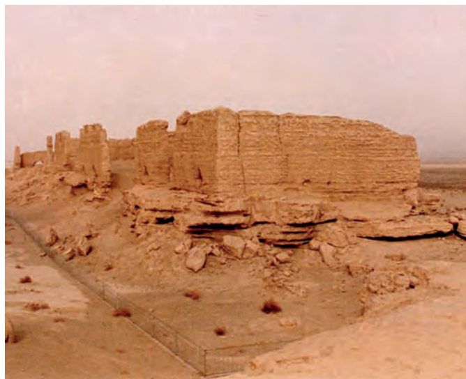
FIGURE 3 Condition of the Hecang Fortress before consolidation.
