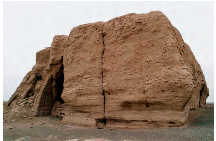
FIGURE 1 Condition of the Yumen Pass before consolidation.
