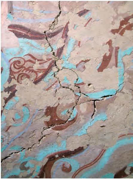
FIGURE 2 Cracks in the painted earthen plaster in cave 85. Photo: S. Rickerby
