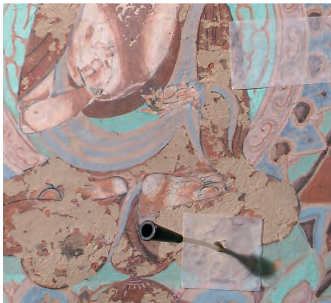
FIGURE 3 A grout catheter placed in an insertion point that has been stabilized with a temporary facing. Photo: S. Rickerby
