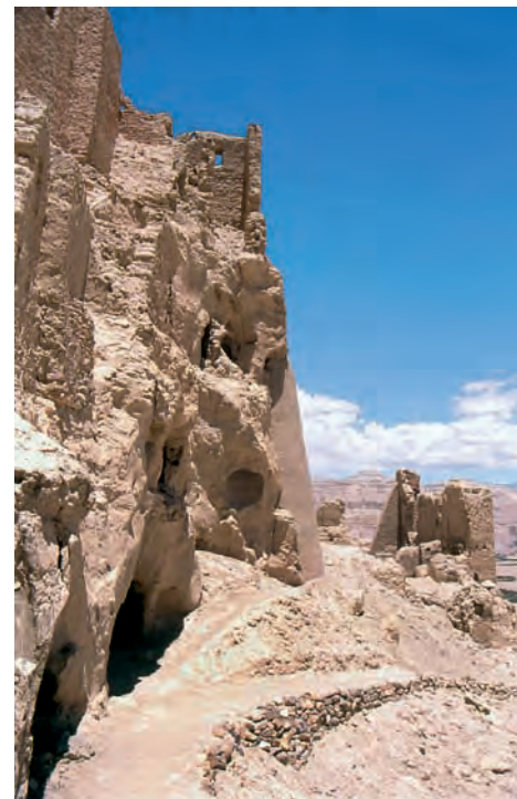
FIGURE 3 Cracking and threatened collapse of earthen architecture.
