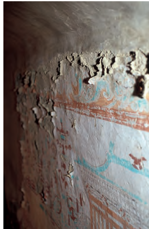
FIGURE 4 Exfoliation, the lifting of paint, ground, and upper plaster layers, apparently exacerbated by treatments for flaking (in the 1970s) using polyvinyl acetate and polyvinyl alcohol fixatives. The continued loss of painting indicates that this problem is ongoing, most notably at the northwest end of the cave.
