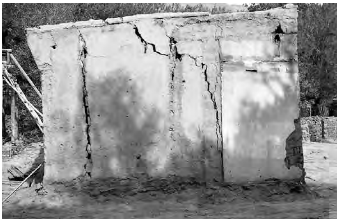
FIGURE 1 Deteriorated north wall of a building in the Upper Temple before restoration.
