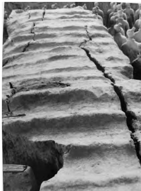
FIGURE 1 Ten-centimeter-wide cracks on the earthen partition wall in pit 1.
