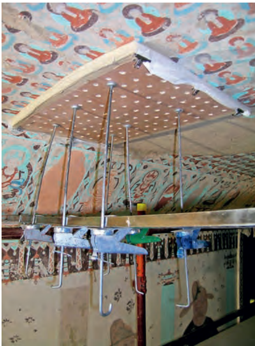
FIGURE 5 A customized press placed against treated plaster for support and to absorb moisture released from the grout. Photo: S. Rickerby
