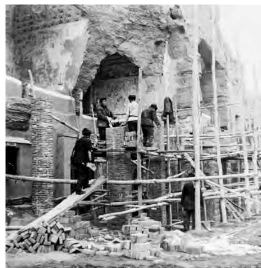
FIGURE 3 Cave 85 during construction of facade and walkways (1957–58). Pillars were built in front of the cave to support a wooden walkway and provide support to the fronts of caves 242 and 243.
