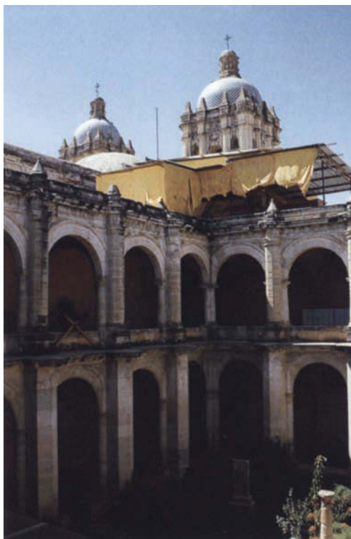
The reconstruction of the roof of the former convent of Santo Domingo. As the museum reconstruction accelerated, massive amounts of particulate dust became an imminent threat to the textile collection. In this urgent situation, all of the textiles were packed in boxes, wrapped in plastic sheeting, and moved to a temporary holding area to protect them from dust while the roof was removed overhead. Photo by K. Klein.
