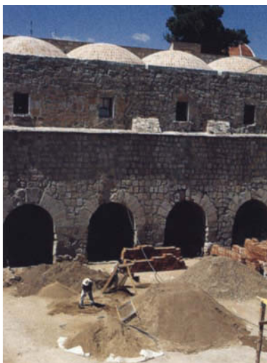
A section of the convent once occupied by the Mexican military. By 1859, under the laws of the Reform promulgated by Benito Juárez, the few friars remaining at the convent were forced to leave. Because of its solid and impenetrable structure, the convent was converted into a military garrison, serving as a prison, a stable, and a depot for military equipment. For many years the convent was occupied by the militaries of either the liberal or the conservative governments of Mexico. Through the mediations of the archbishop of Oaxaca, in 1895 the church and a small annex of the convent were returned to the Dominicans. Photo by K. Klein.
