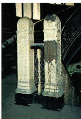
FIGURE 6. The Rookery, oriel stair newel posts, above, overpainted condition before restoration.
