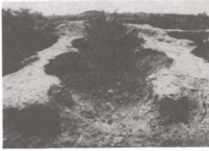
Figure 10. A view of the "Archives" in Seleucia. The top of the walls was capped with soil-cement, which did not prove to be effective, since there was formation of water pools at the bases of the walls.
