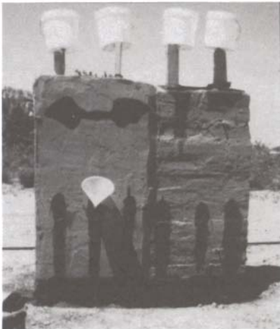
Figure 6. Photograph showing adobe test wall being treated with chemical consolidant using bulk infiltration technique.
