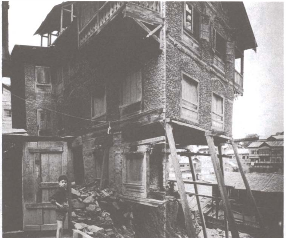
Above right: A Taq system house undermined by the river shows the remarkable flexibility and strength of this timber/masonry system (and the fearlessness of the workers.)
