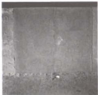
Very little erosion.
