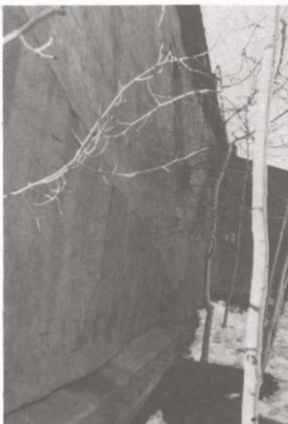
Figure 8 Distressed Cement Stucco Holy Trinity Church Arroyo Seco, New Mexico
