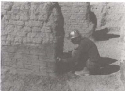
Workman contouring new adobe bricks to fit profile of historic wall, 1974. New Mexico State Monuments.
