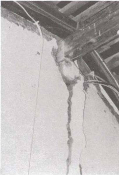
Figure 8. Damage from cocina ridge beam, the Castro Adobe, 1990
