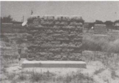
Fig. 4 Example of test wall constructed with concrete wainscot installed along the base.
