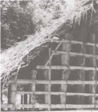
Figure 2. A part of the timber skeleton of a wattle and daub house showing a column supporting the roof, vertical 'core columns' and horizontal bamboo splinters.
