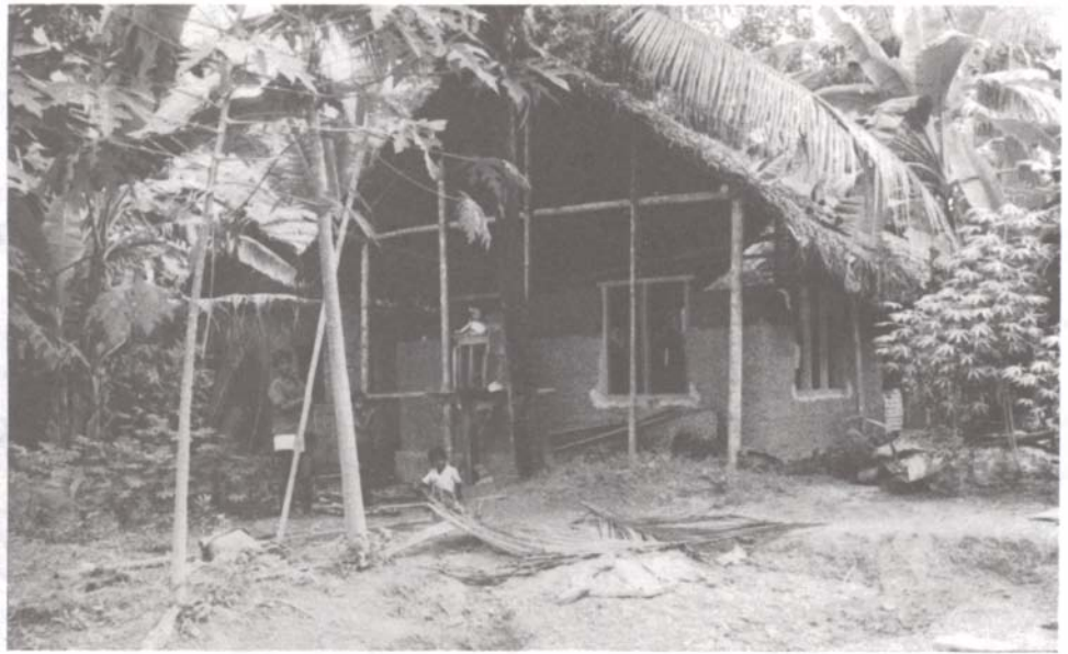
Figure 5. A house with rammed earth-walls, under construction; note the temporary roof standing on timber supports.
