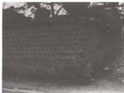
Fig. 1: Wall with "mole-do" base and adobe masonry. Tiradentes, Minas Gerais. Photo: Lima.
