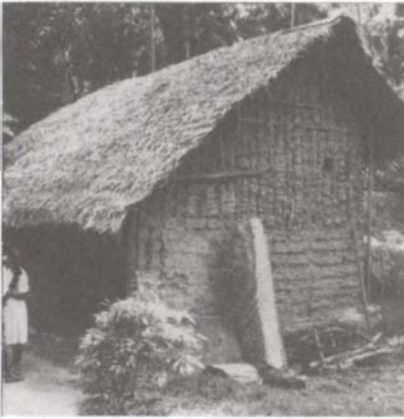
Figure 12. The exposed timber skeleton, of a wattle and daub wall, after the loss of the second coating of mud.
