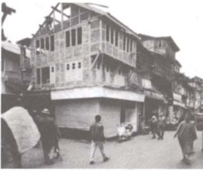
A Dhajji Dewari house being reconstructed using the traditional materials, including mud mortar. All of the exterior walls were reconstructed while the family continued to live in the house.
