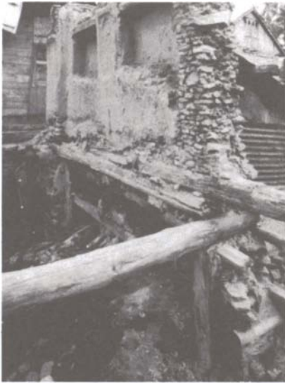
Above: A house in ruins shows the timbers imbedded at each floor level in the Taq System masonry wall.
