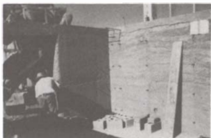
Figure 4. Exterior 60-cm-thick rammed-earth wall of home under construction by Soledad Canyon Earth Builders, Mesilla, New Mexico.
