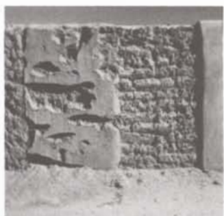
Very serious erosion.
