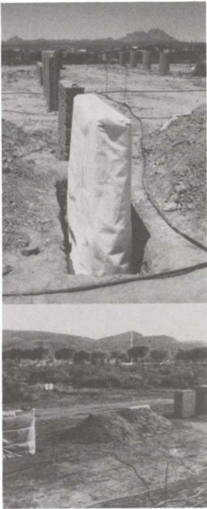
Figure 18. Photographs showing geotextile-covered and uncovered walls (#43, 44, respectively) a) prior to burial, and b) after burial.
