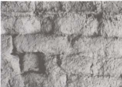
Figure 16. View of the same wall in 1989. The bricks on the top are washed away from the rain, and the material ran over the lower, consolidated part.
