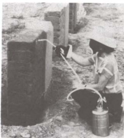
Figure 4. Photograph showing chemical consolidant being applied to adobe test wall by spraying.
