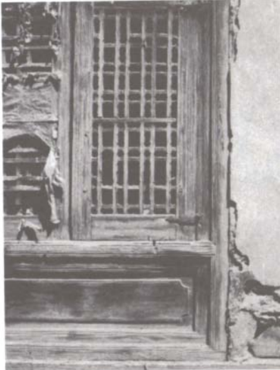
The Jalli shutters showing, on the left, the remains of the paper attached for winter protection.
