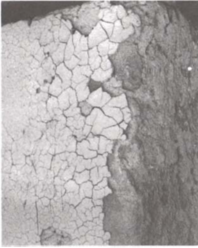
Figure 11. The cracked kaoling coating falling off a mud wall.
