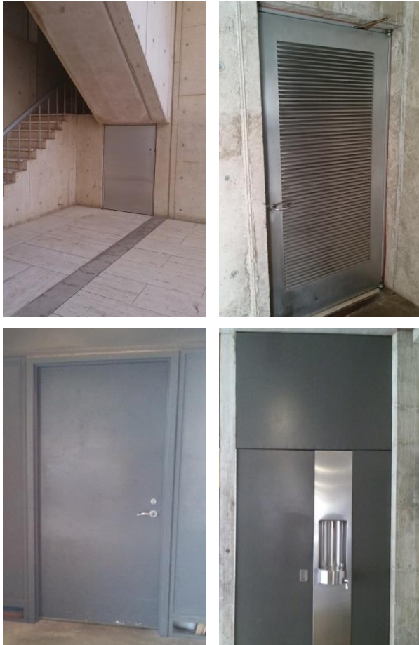
Top left: Kahn-designed flush stainless steel door. Top right: Kahn-designed louvered door. Bottom left: Post-Kahn introduction of painted hollow flush metal door. Bottom right: Kahn-designed painted steel paneling and polished steel drinking fountain.
