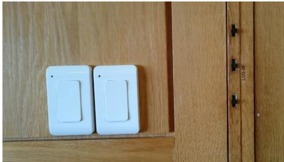
Top: Ad-hoc plethora of cabling in offices. Bottom: Intrusive addition of new switches (left); original switches integrated with millwork (right).
