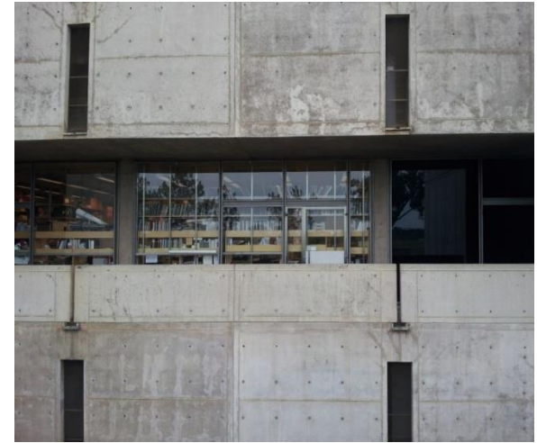
Typical tripartite stainless steel window wall altered to accommodate more than one entrance into a typical laboratory bay.
