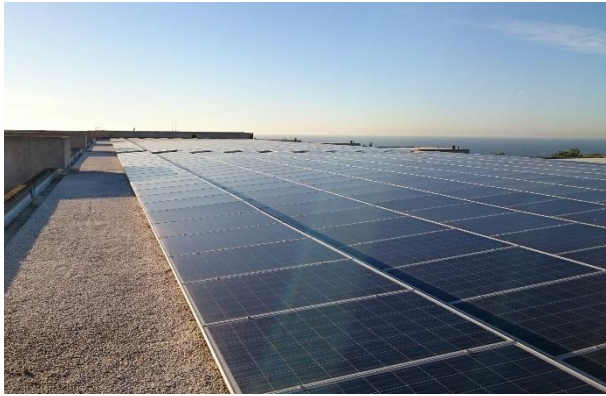
Roof solar panels.
