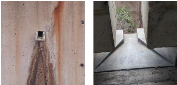
Left: Kahn's lead scupper to roof garden. Right: Kahn's lead scupper to laboratories.
