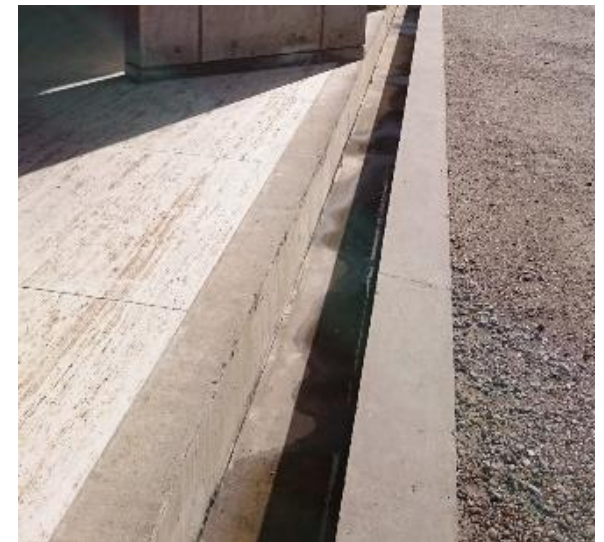
Top: Cascade and moat infilled by later metal duct is intrusive Bottom: Moat to arcades of office wings.
