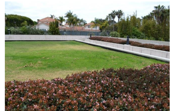
Top: View of the northern lawn panel. Bottom: View of the undulating south lawn, the turf exhibiting poor growth, and the subsidence evident along the wall.
