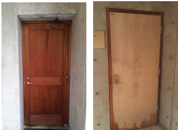
Left: Teak door and hardware by Kahn to North Study Towers. Right: Plywood door were installed at the South Study Towers due to economic cut backs.
