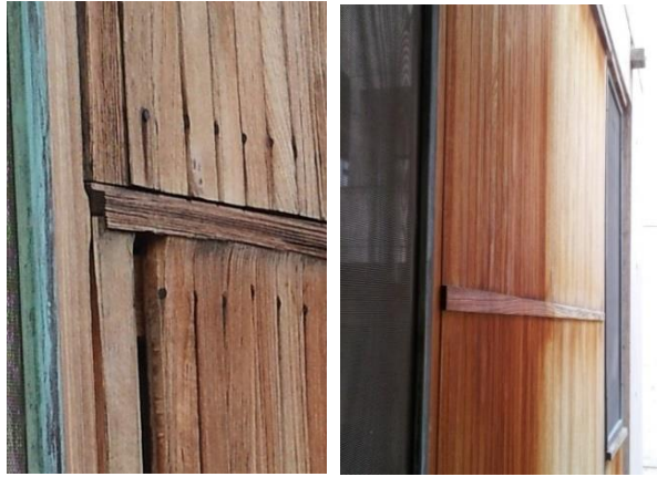
Left: erosion of water tables by erosion: exposure of secret nails and loss of siding. Right: Impact of differential weathering on teak siding. At left, the non-original red-colored varnish remains, while at right, the teak surface is exposed.
