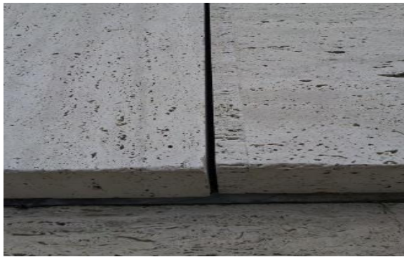
Top: Minor fractures in travertine do not warrant replacement. Bottom: Careful attention to detail required when repairing travertine.
