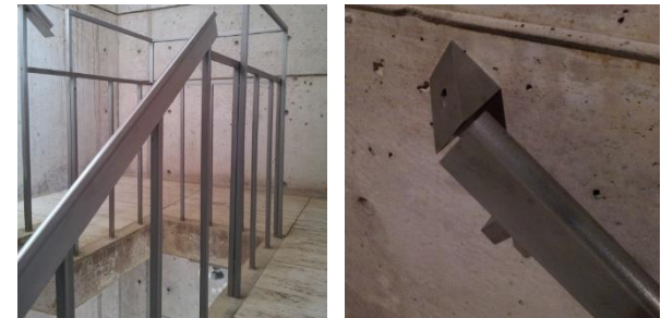
Left: Kahn’s original stainless steel railings and extruded stainless steel handrail and the 1972 additional safety railings. Right: Kahn’s end detail to wall rails.
