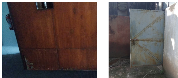
Fig. 159: Worn door corners (L); Ad hoc additions (R)
