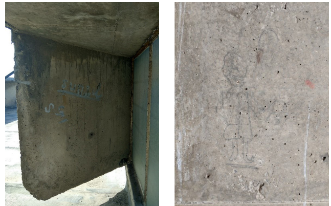
Fig. 189: Graffiti in paint on fins at terrace level (L); on external columns (R)
