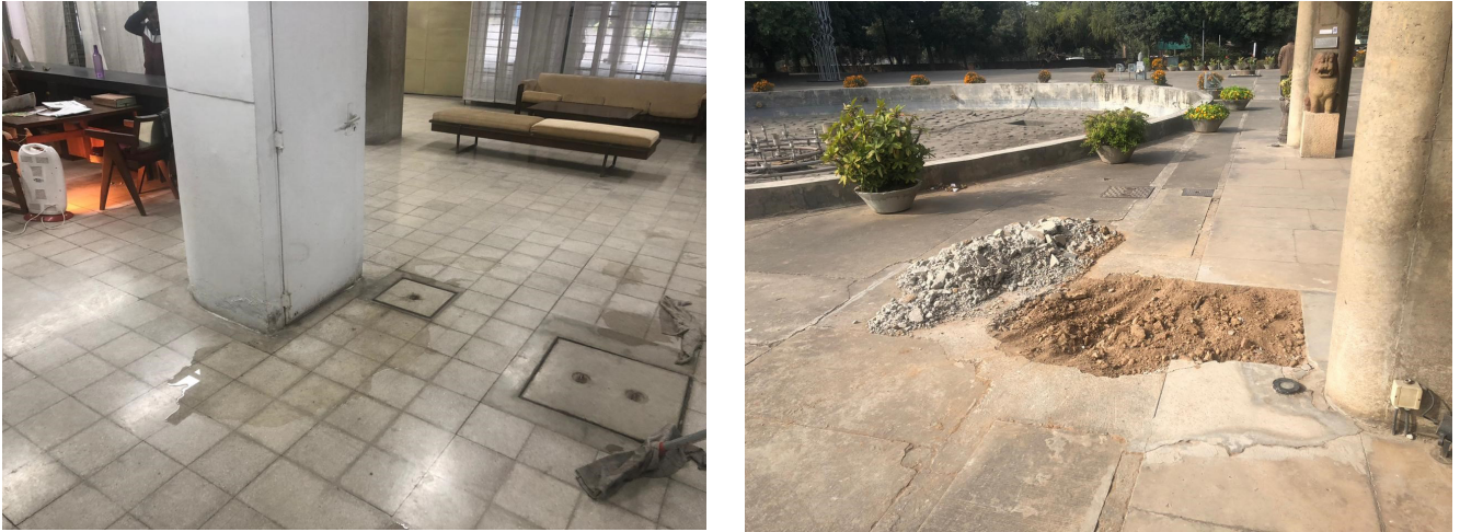
Fig. 186: Water leakage due to damaged pipework under floor of entrance lobby (L); Main water supply has been temporarily blocked to check the leakage (R)
