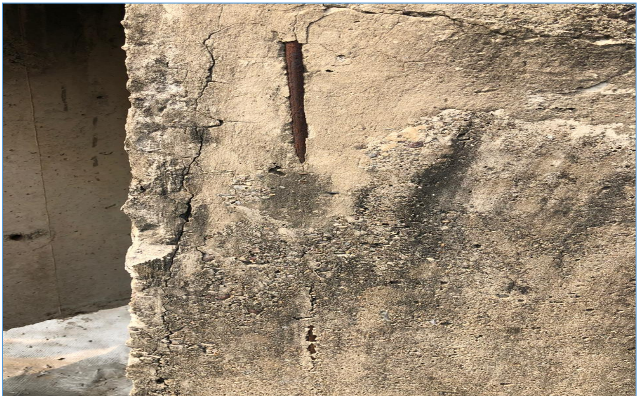
Figure 8 Exposed reinforcement bar leads to corrosion of reinforcement, resulting in cracks & spalling of concrete.
