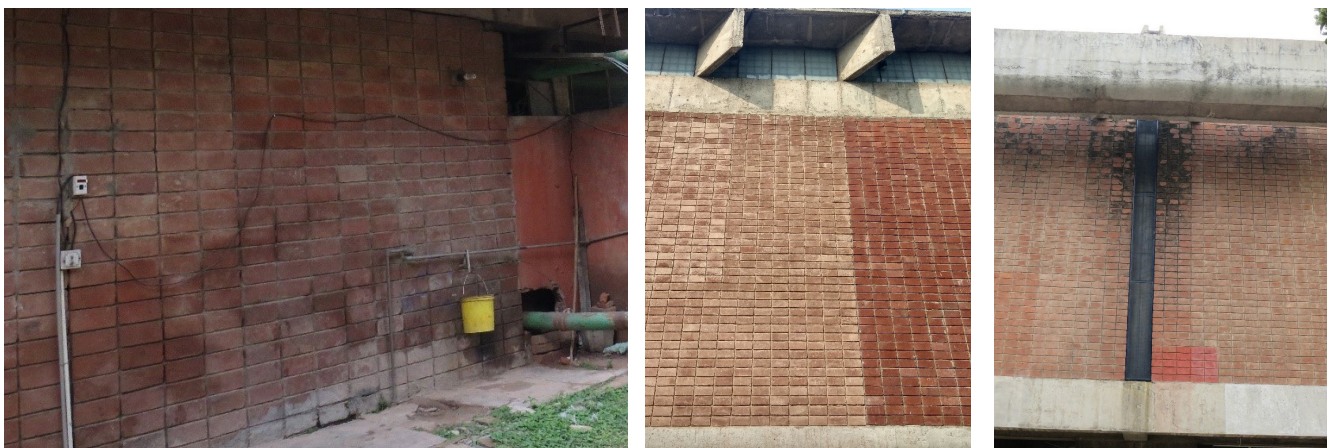
Fig. 145: Brickwork damaged due to water seepage (L); Discoloration of replaced bricks (C); Algal growth on brick tile surface under gargoyle (R)
