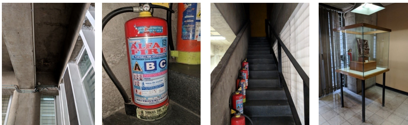
Fig. 187: (L-R) Area of past incident; Type B extinguisher; Units stored on the staircase; Fire extinguishers hidden away behind exhibits
