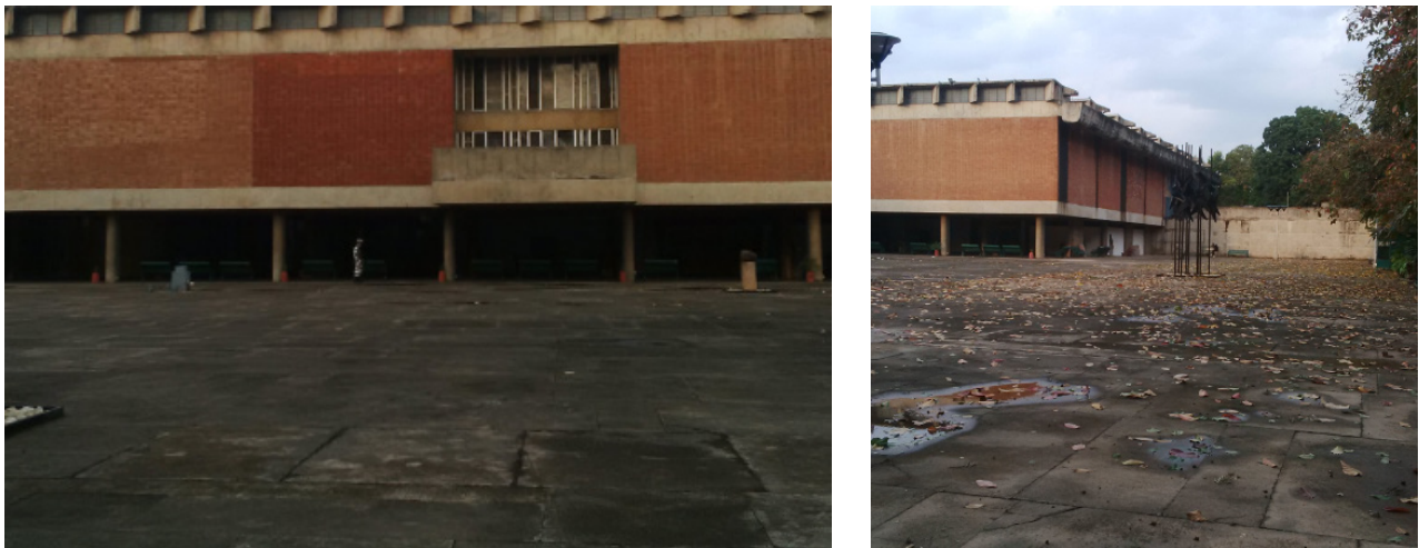
Fig. 128: Condition of piazza flooring- water-logging at places, discoloration of concrete surface
