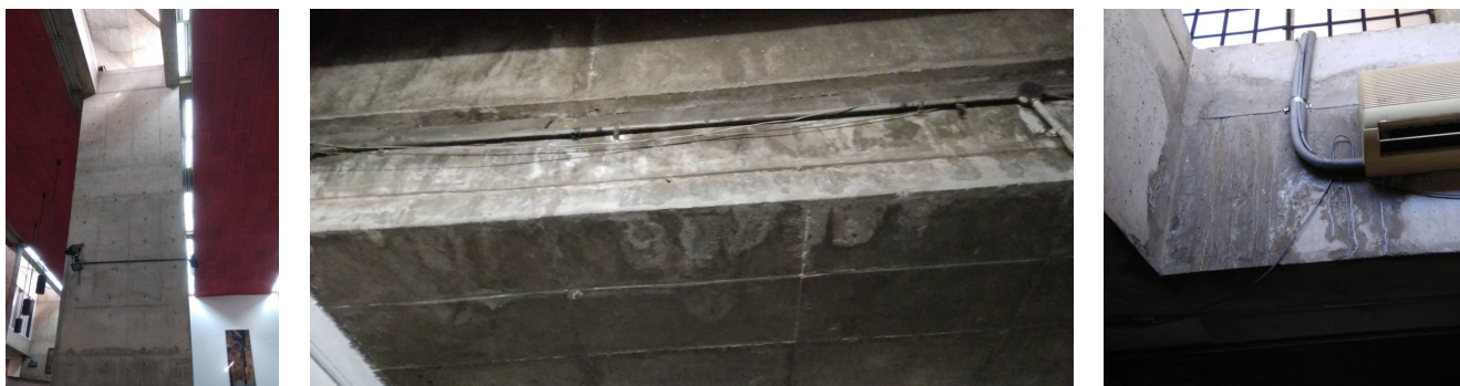
Fig. 149: Water seepage from clerestory windows (L); Failing air conditioning pipes (C)(R)
