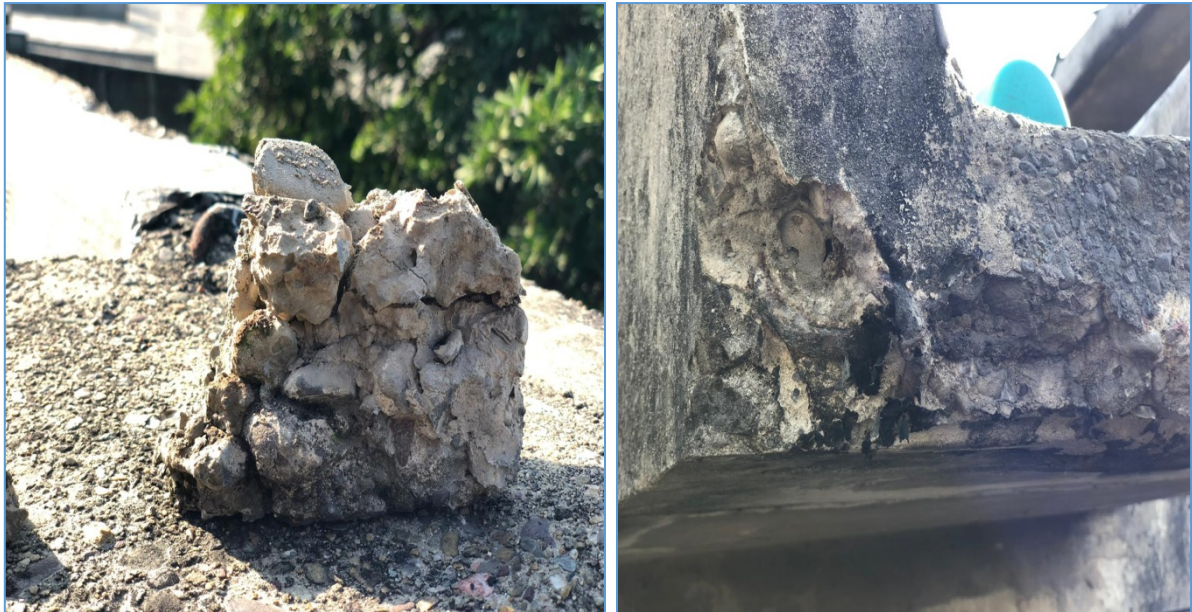
Figure 7 loose concrete fallen down just by light tamping with hammer
