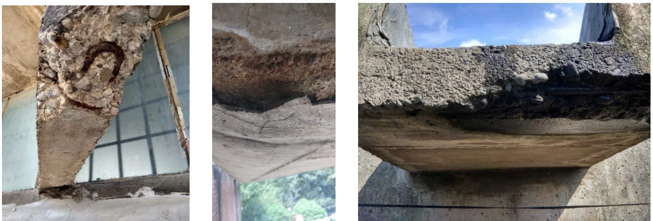
Fig. 136: Spalling leading to loss of material and exposed rebars along the outer edges of fins(L); Concrete spall at the underside of concrete drains (C)
