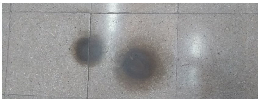
Fig. 154: Tile damage due to water dripping from roof
