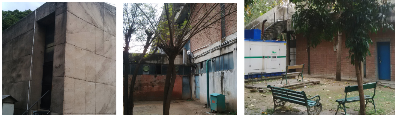
Fig. 134: Air Conditioning outdoor units at the rear side of the auditorium (L); Trees have been heavily pruned in the utility areas (C); The DG set within a rather unkempt landscape, hidden from the public view, but with garden benches (R)
