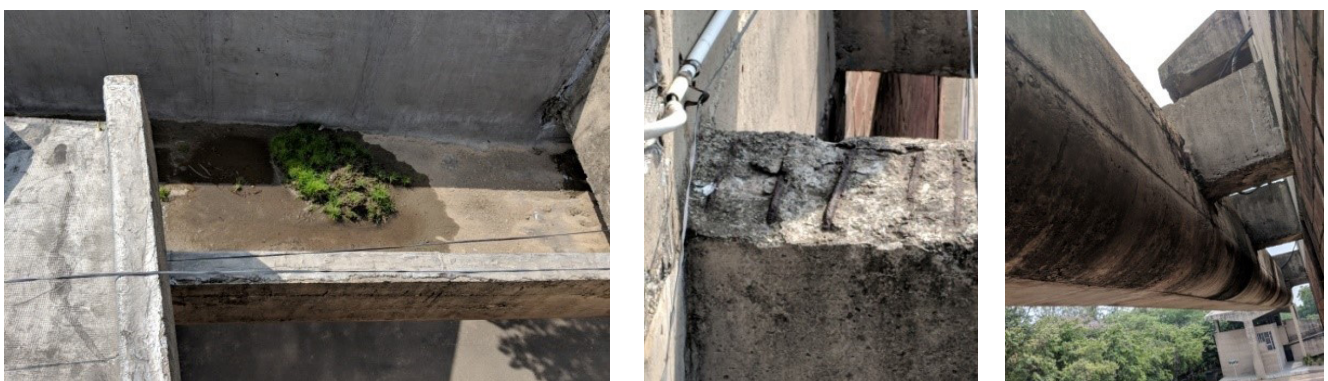
Fig. 190: Vegetation growth in concrete duct (L); Exposed reinforcement bars and major cracks seen on beams connecting the concrete drains to the building (C)(R)
