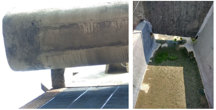
Fig. 141: Failing patch repairs (L); Water stagnation inducing vegetation growth within concrete drain (R)
