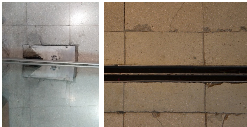
Fig. 153: Modern alterations damaging original terrazzo floor tiles
