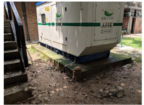
Fig. 199: Water logging at the base of electrical transformer
