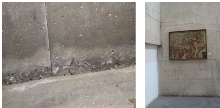
Fig. 148: Discoloration due to daily swabbing
