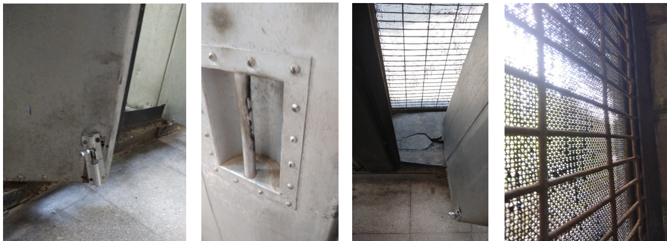
Fig. 160: Damaged door fixtures, concrete sill and rusting grills.
