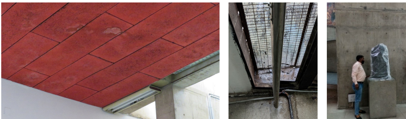
Fig. 192: Damp stains on false ceiling (L); Water seepage through aerators (C); Sculpture wrapped to protect from seepage (R)
