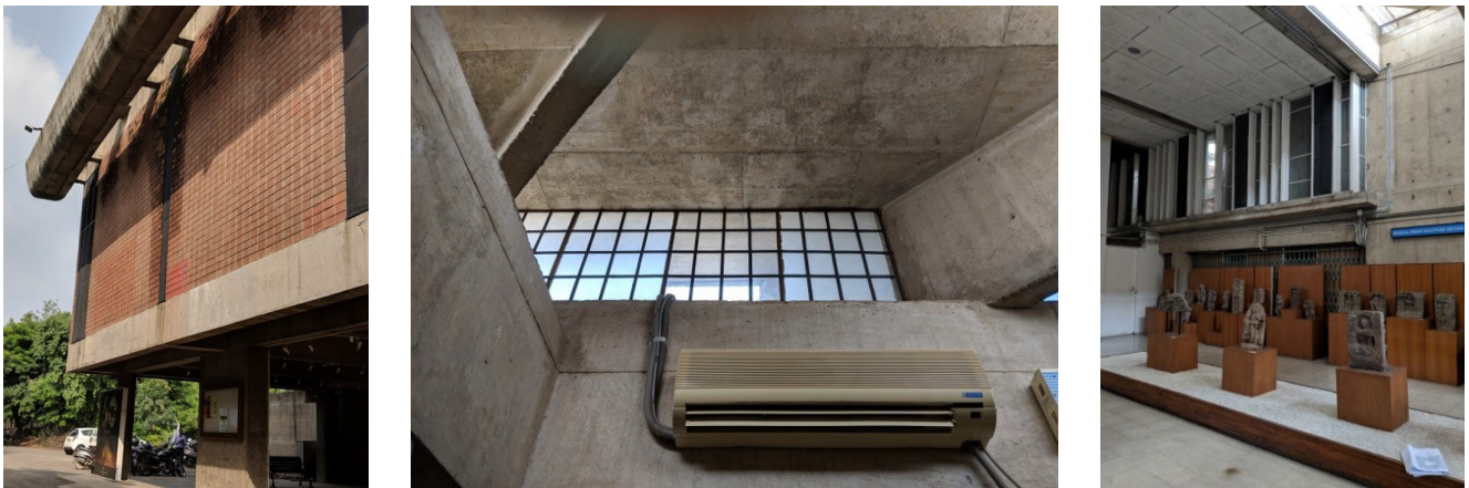
Fig. 191: Dampness seen on external wall (L); Discoloration of ceiling due to water seepage (C); Marks on interior floor tiles due to water dripping from the roof in the past (R)
