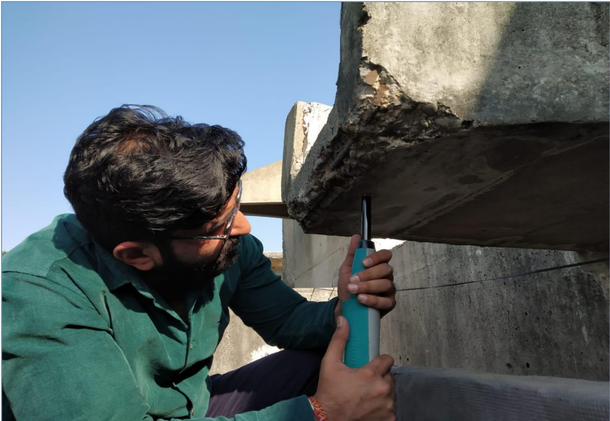
Figure 5 Rebound hammer test of extended channel for pouring of rain water from roofslab into the Gargwell (rainwater drain)
