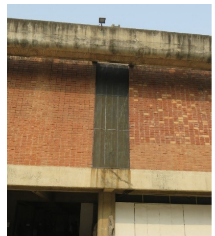
Fig. 139: Rust stains on concrete beam due to water washing over rusted metal mesh at the window openings
