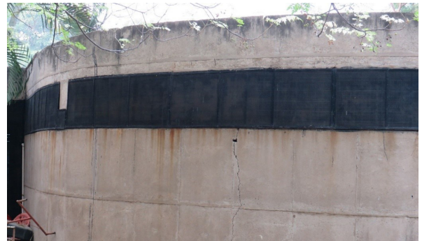
Fig. 135: Cracks due to repairs made in the interior of the temporary exhibition gallery
