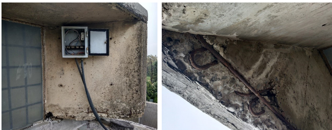
Fig. 137: Exposed rebars of terrace elements
