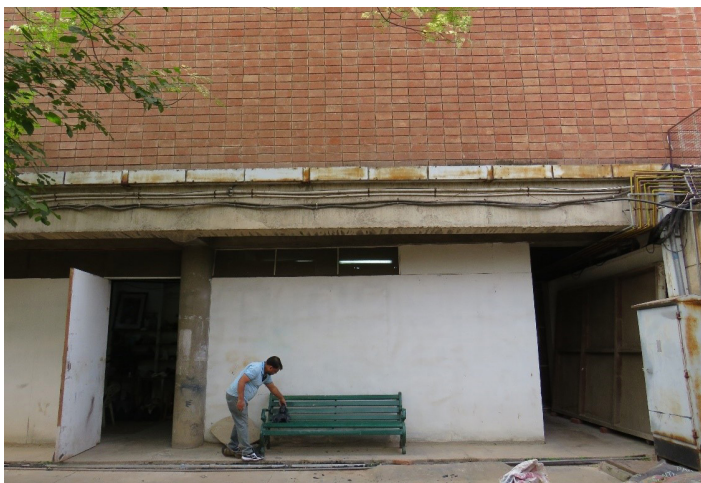
Fig. 182: Objects Exposed electrical wiring and conduit casing disfiguring the building façade
