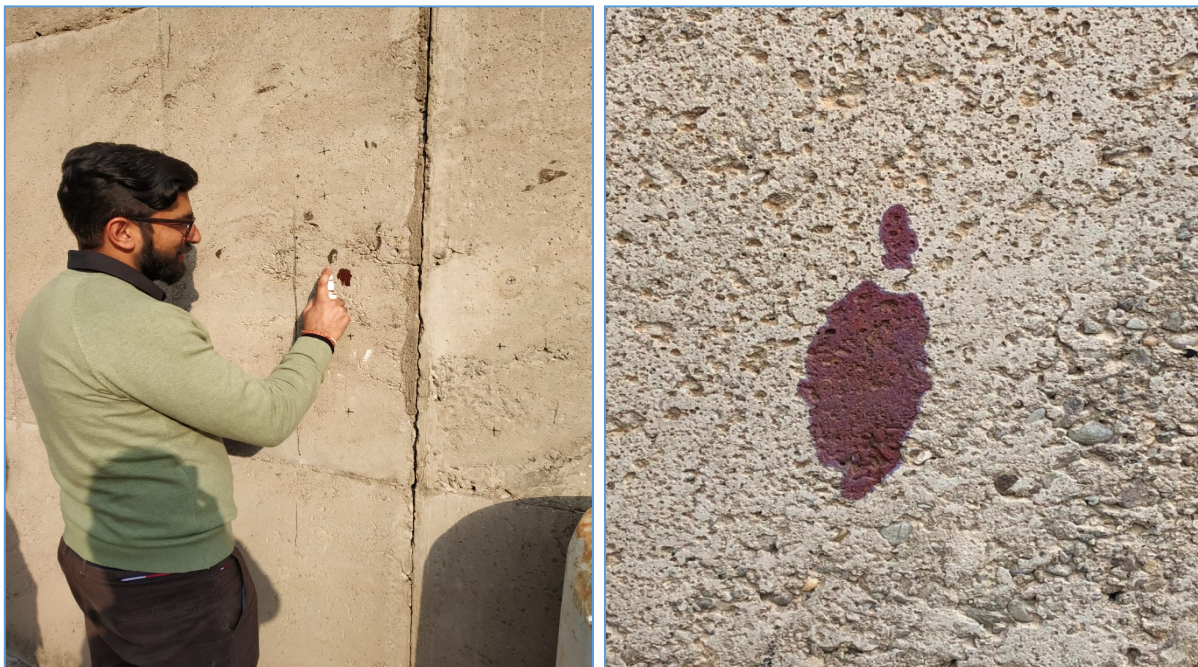
Figure 6 Carbonation test showing red colour over the concrete surface.
