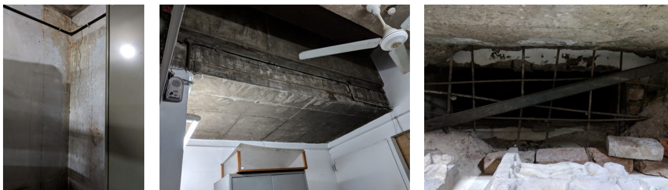
Fig. 197: Damp walls and ceiling in storage areas (L)(C); Unfinished construction between two storage areas (R)
