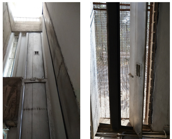
Fig. 69: Centrally pivoting ventilator shutters.
