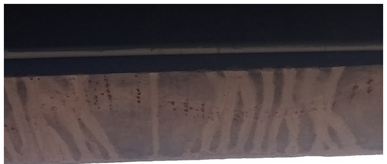
Fig. 143: Rust staining and exposed rebars due to loss of concrete cover
