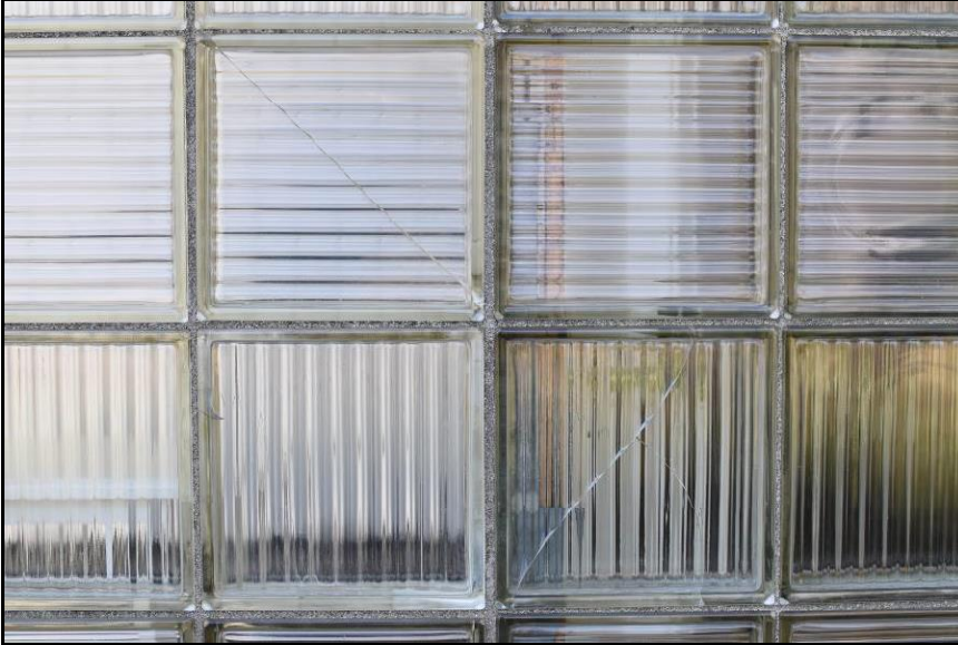
Figure 11. Typical cracks in glass block units.
