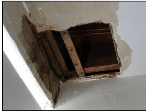
Nominal 2" framing stock as in the first floor ceiling due to a radiator leak
