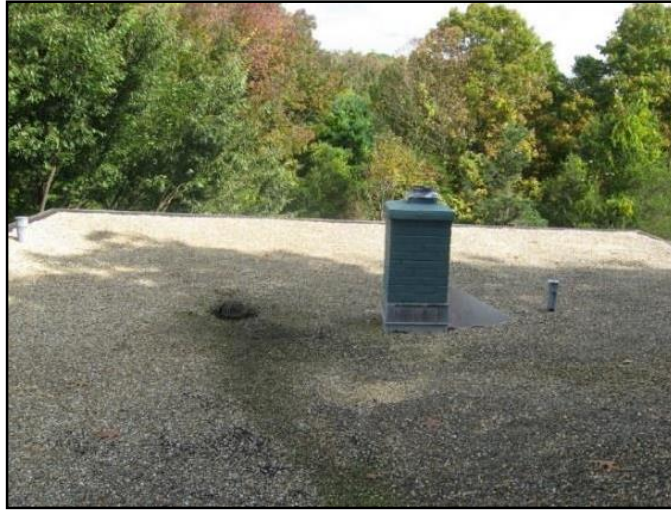
Main body of roof with center chimney, vent stack (right) and roof drain (left)
