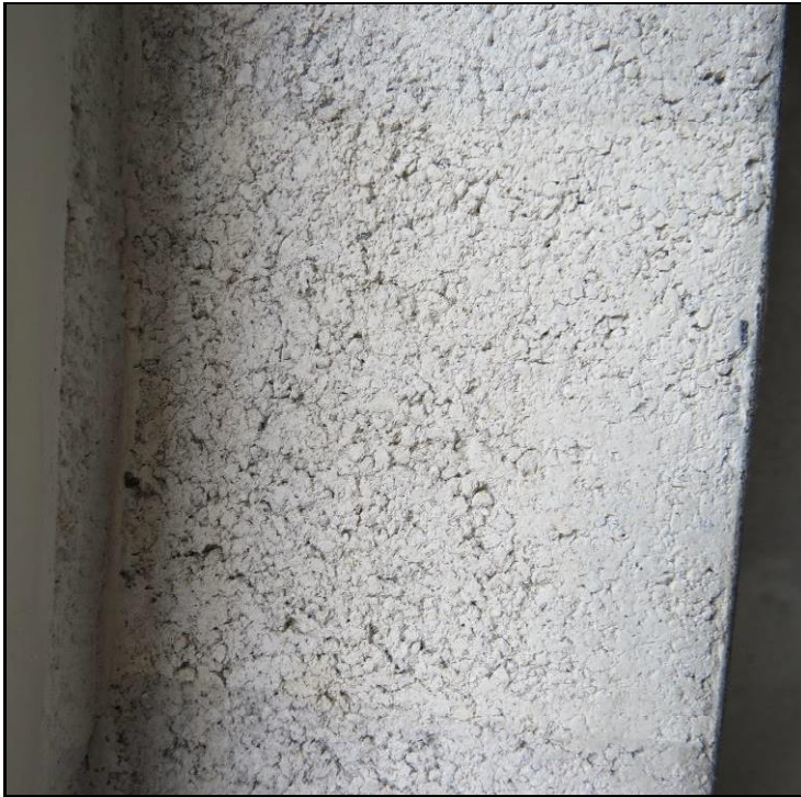
Figure 27. ABR Type A test patch, post-treatment.
