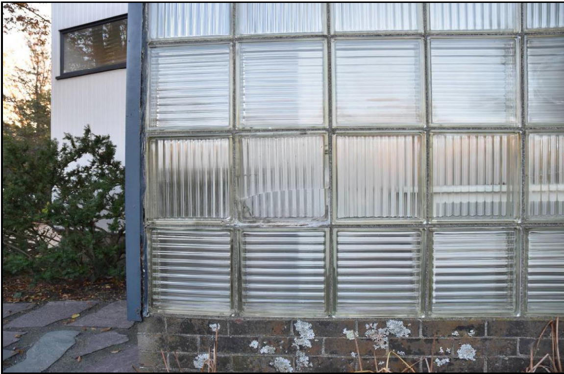
Figure 15. The lower portion of a Block H2 (second course from bottom, 2 nd block from left) has broken away as a result of stress cracking exacerbated by freezing moisture. Note the displacement of the metal channel (left of glass block) caused by corrosion.
