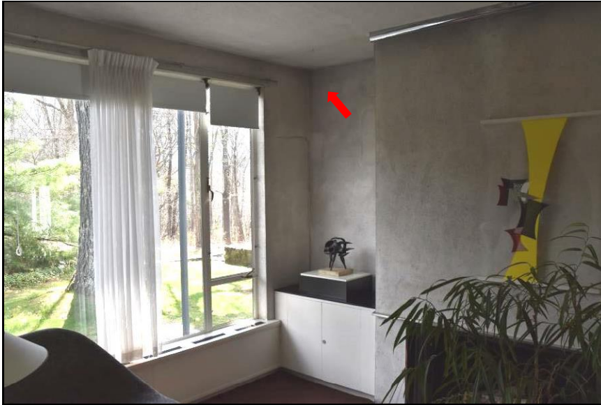
Figure 24. Location of abrasive cleaning tests (red arrow) on west living room wall.
