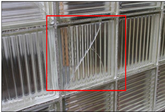
Typical intact fracture of glass block
