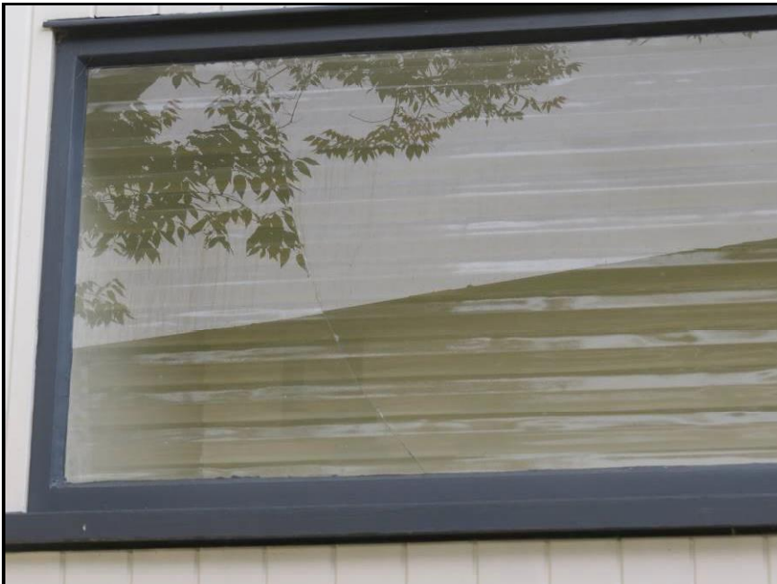
Figure 9. A single stress crack seen in Window 111.
