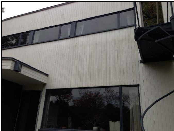
Excessive mildew build up on north elevation
