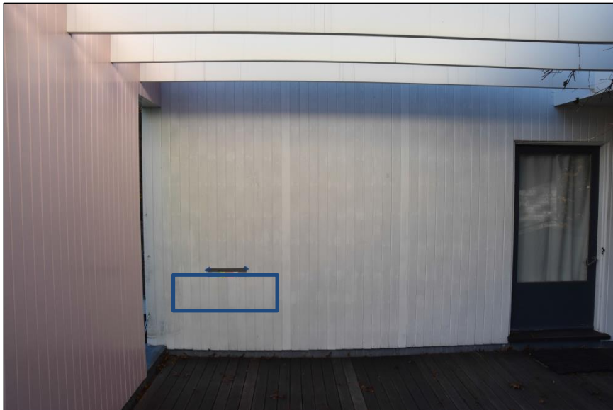
Figure 13. Cleaning test location on west elevation of the second story roof deck.
