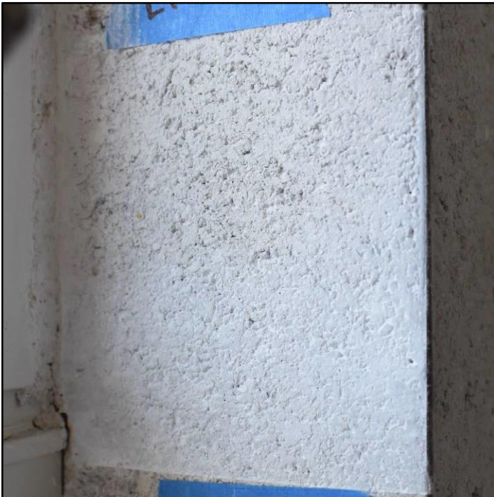
Figure 40. Brushed-on acrylic-modified lime putty limewash test patch with one (above) and two (below) coats.
