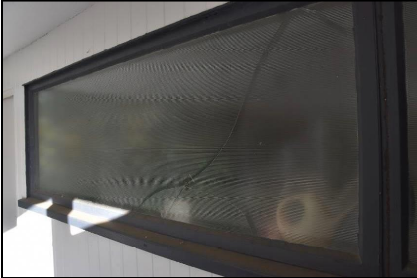
Figure 6. Stress/impact related damage in fixed-pane of Window 102.
