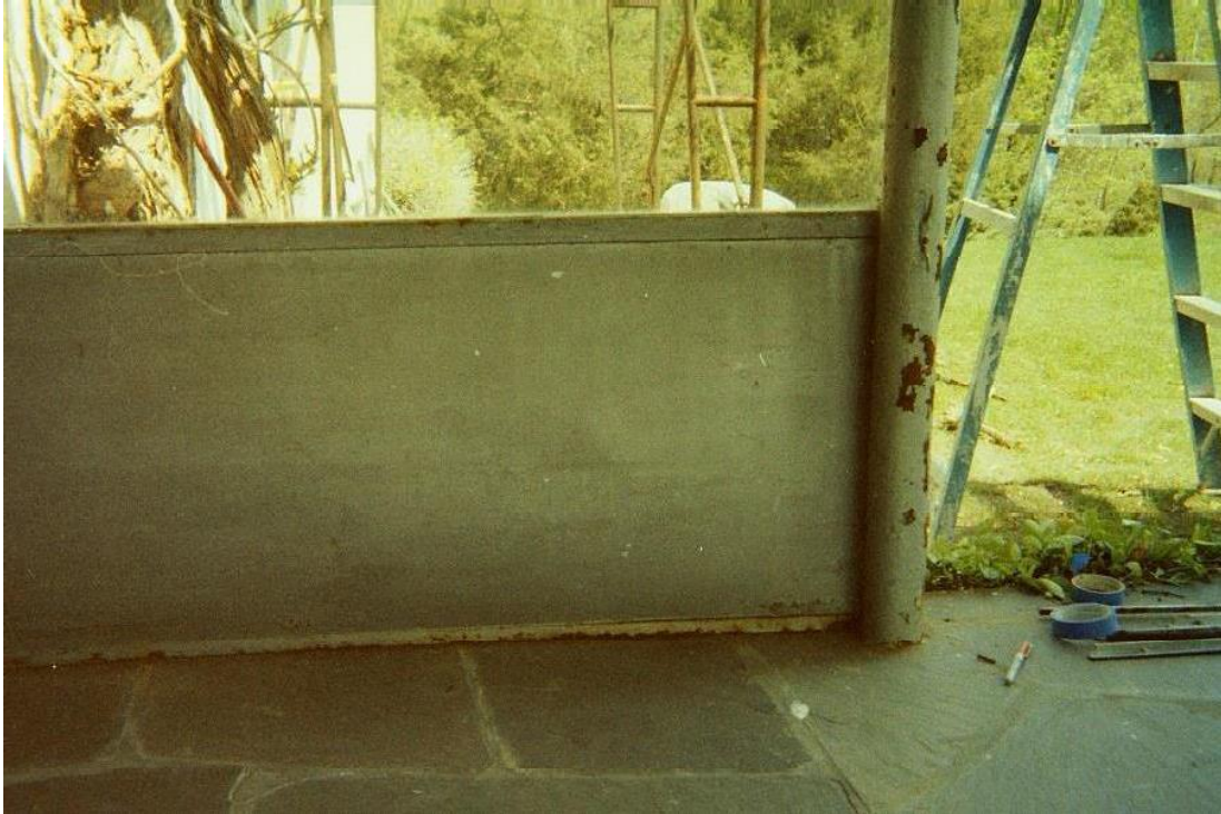
Figure 3: Damaged steel column near porch, 2001 Historic New England Property Care Binders
