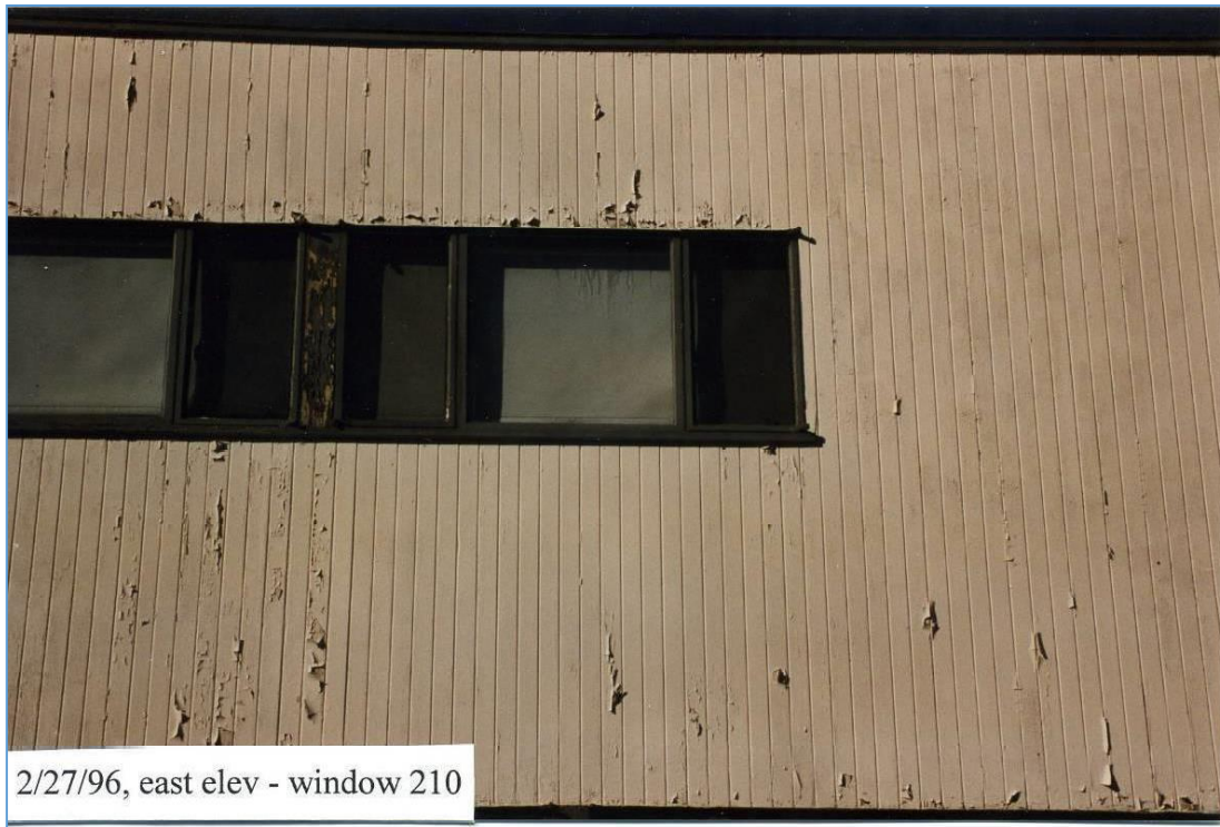
Figure 4: Siding condition, 1996 Historic New England, Property Care Binders
