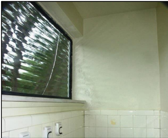
Example of broken specialty glass
