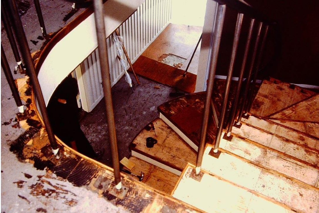
Figure 2: Stair and hall during cork floor replacement, 1988 Historic New England Archives, Binder of Slides
