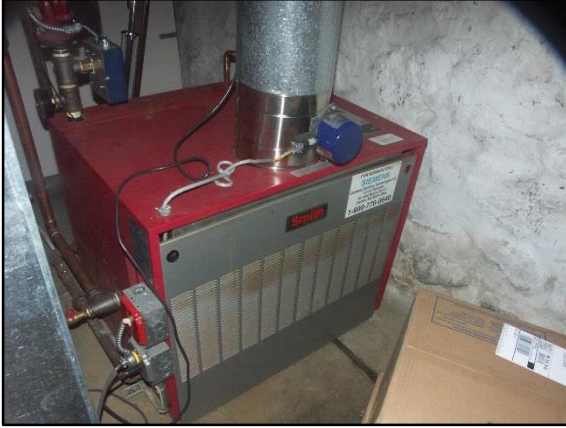
Gas fired boiler
