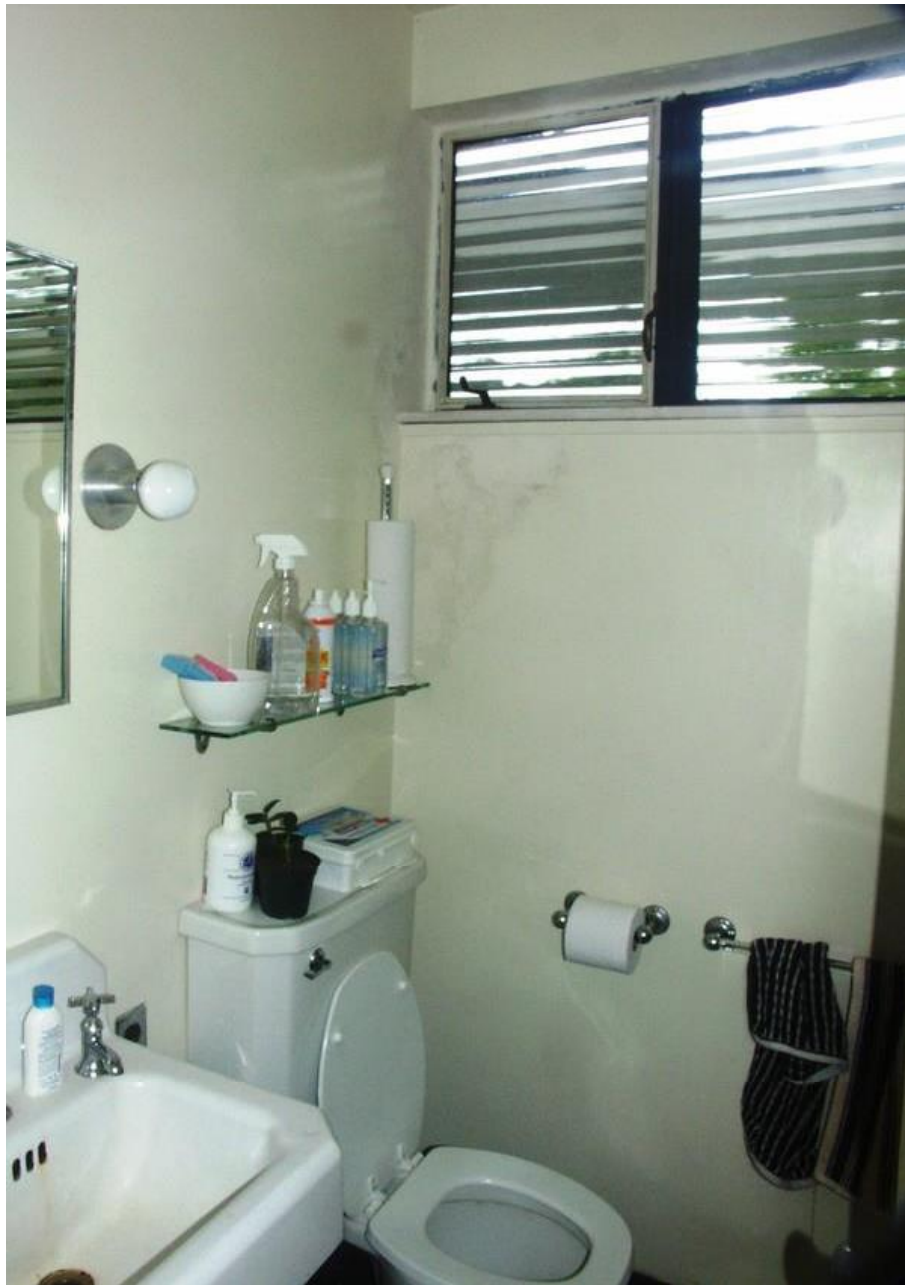
Figure 4: Stained bathroom walls, 2009 RS ID #56596
