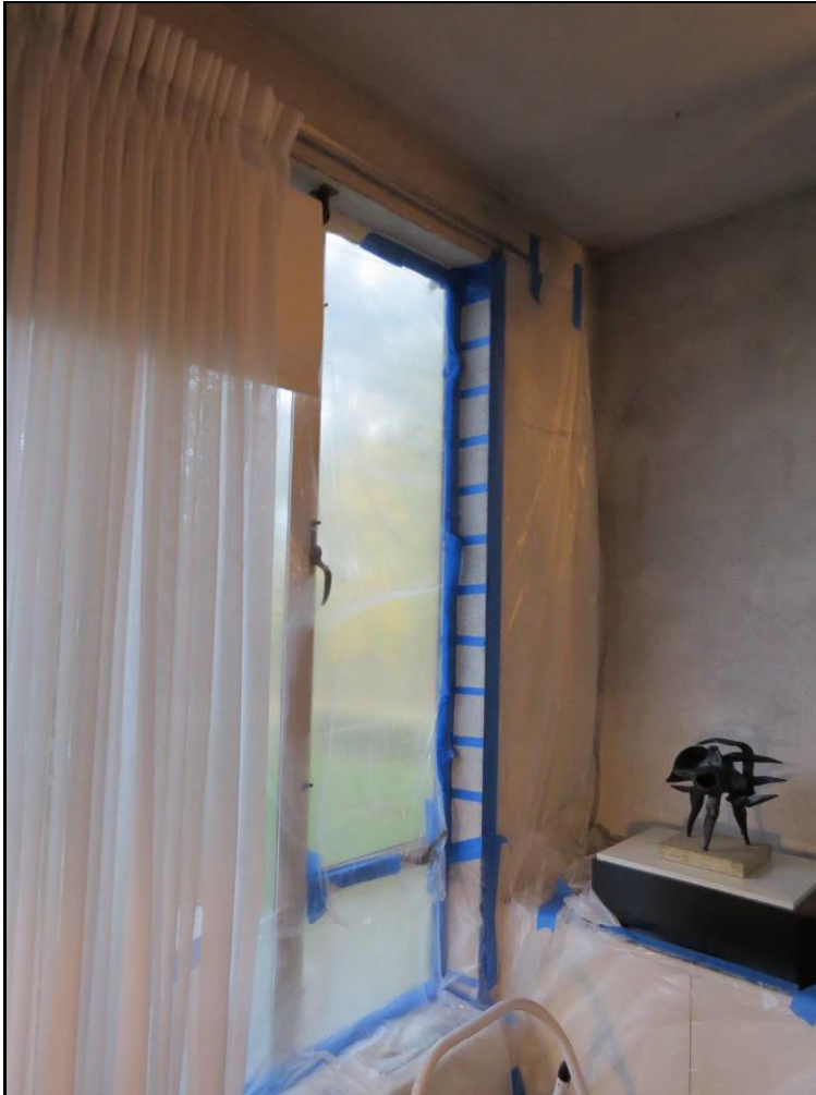
Figure 23. Location of cleaning test patches (marked in blue tape) on window return in living room.
