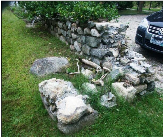
Wall damage at top of driveway
