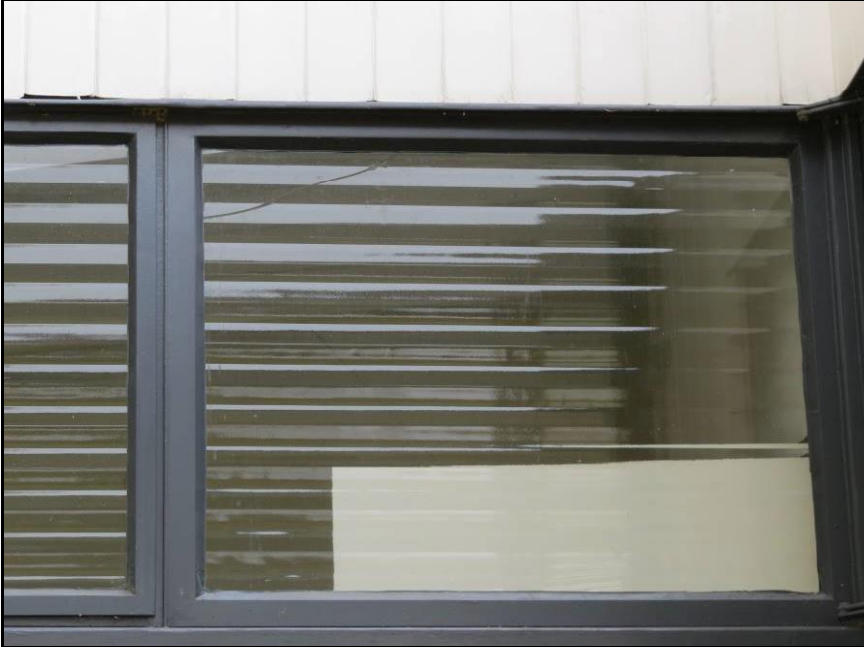
Figure 8. A single stress crack seen in Window 110.
