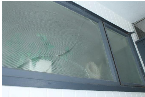
Figure 7: Crack in ribbed glass on south elevation, 2015 RS ID #277155
