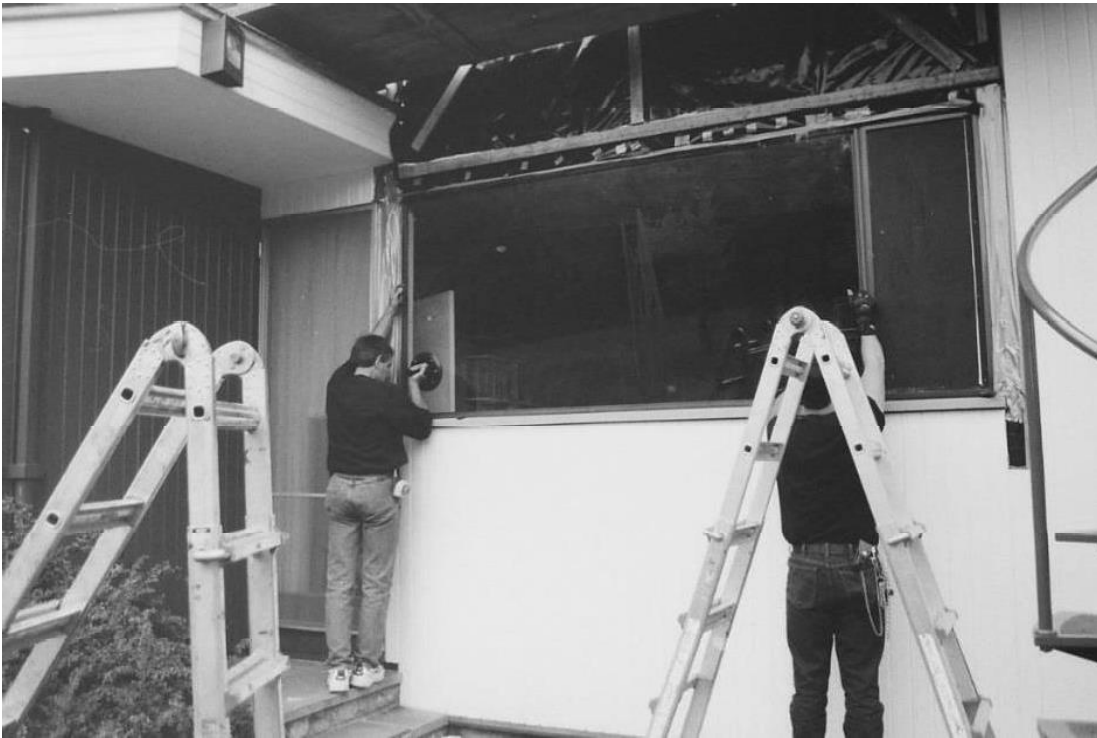
Figure 7: Steel window restoration work, 1997 Historic New England Property Care Binder, Lyman Estate
