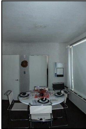
Dining Room view showing ceiling discoloration and lighting fixture
