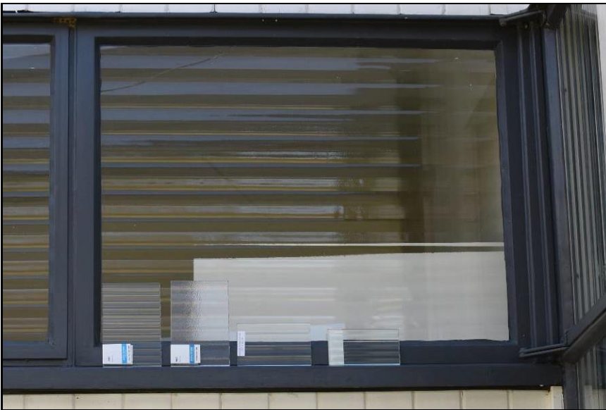
Figure 18. Samples of replacement glass compared to original Louvrex glass in Window 110 (north elevation). Samples (left to right): AGC “Flutes” Clear Pattern, AGC “Textured Flutex”, Gray Glass “1-inch Fluted”, Bendheim’s JBCO-35.
