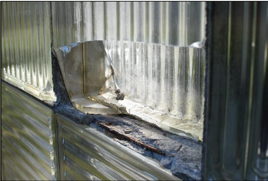
Figure 12. Block H2 exhibiting extensive cracks, losses, and exposed corroding metal joint reinforcement.
