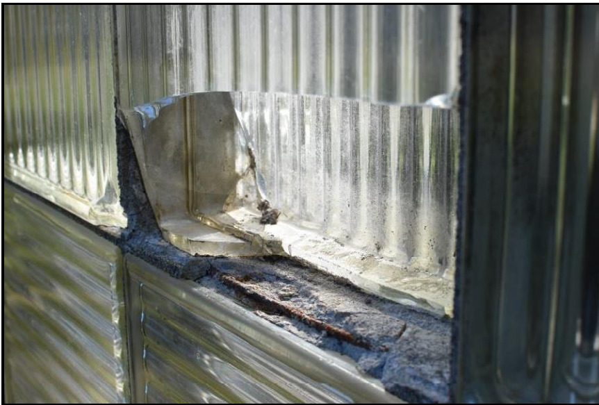
Figure 12. Block H2 exhibiting extensive cracks, losses, and exposed corroding metal joint reinforcement.
