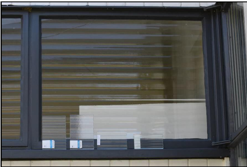
Figure 18. Samples of replacement glass compared to original Louvrex glass in Window 110 (north elevation). Samples (left to right): AGC “Flutes” Clear Pattern, AGC “Textured Flutex”, Gray Glass “1-inch Fluted”, Bendheim’s JBCO-35.
