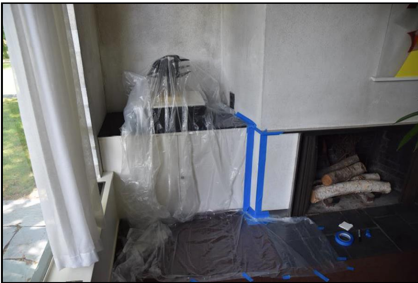
Figure 26. Location of pigmented limewash test patch (outlined in blue tape) adjacent to living room fireplace.
