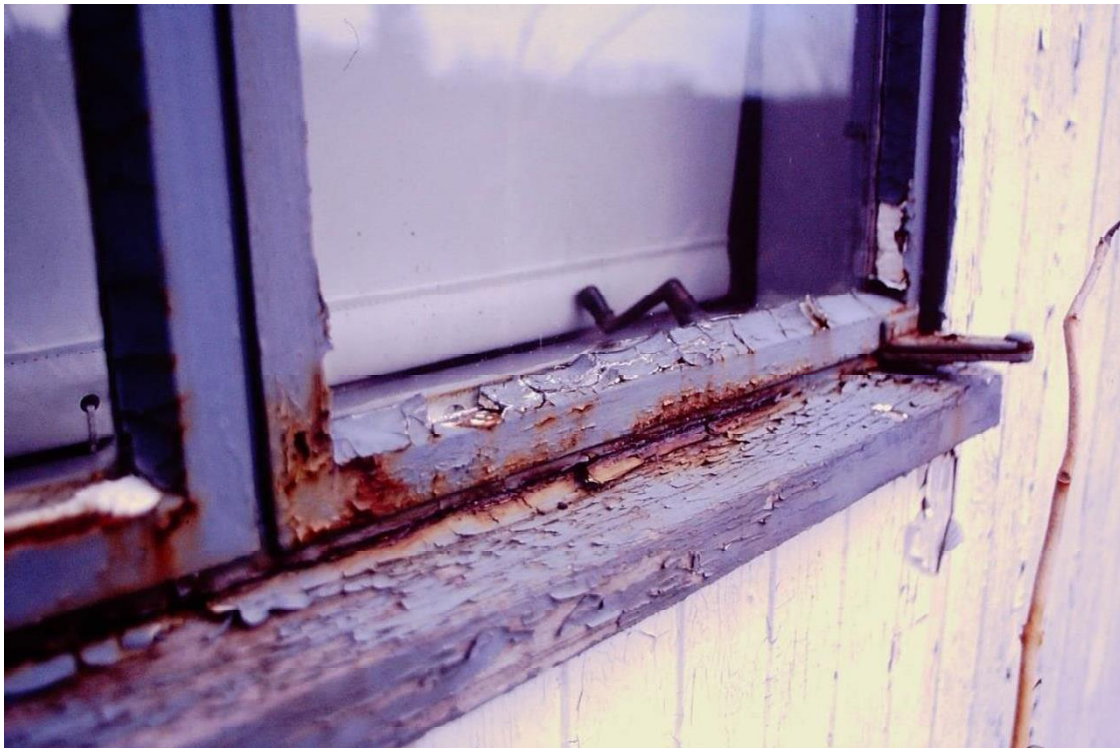
Figure 5: Rust on the south elevation master bedroom window, 1990 Historic New England Property Care Binder, Lyman Estate
