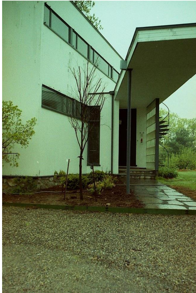
Figure 7: Flagstones under marquee and driveway gravel, 1989 Historic New England Property Care Binders
