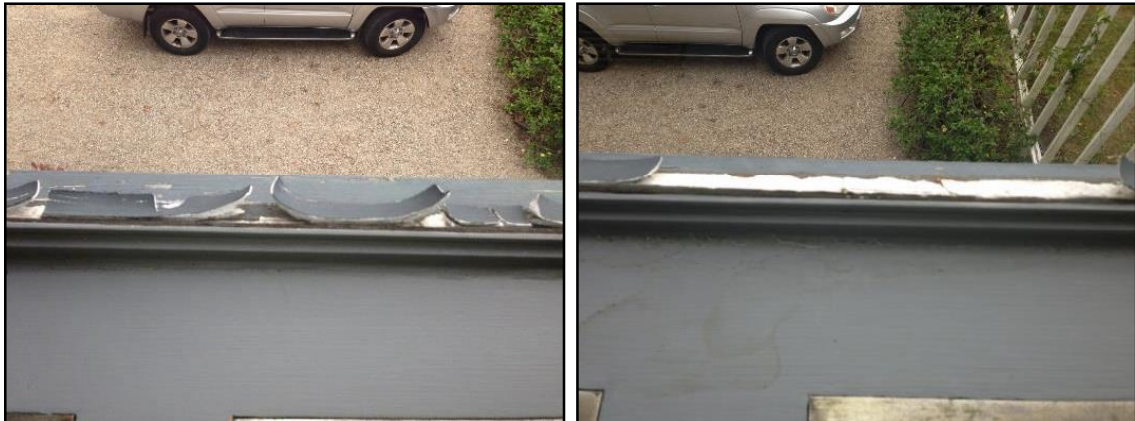
Typical glazing failure issues on east elevation - 2013
