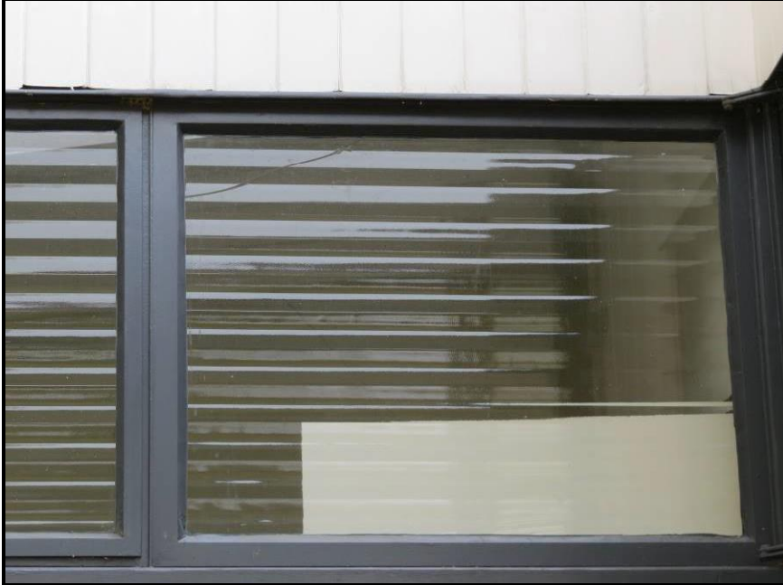
Figure 8. A single stress crack seen in Window 110.
