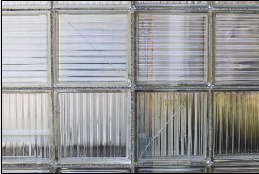
Figure 11. Typical cracks in glass block units.
