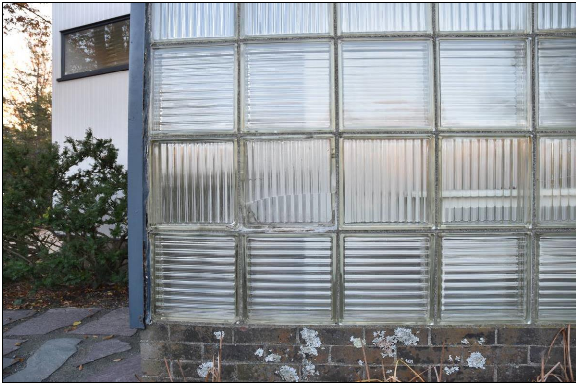
Figure 15. The lower portion of a Block H2 (second course from bottom, 2 nd block from left) has broken away as a result of stress cracking exacerbated by freezing moisture. Note the displacement of the metal channel (left of glass block) caused by corrosion.
