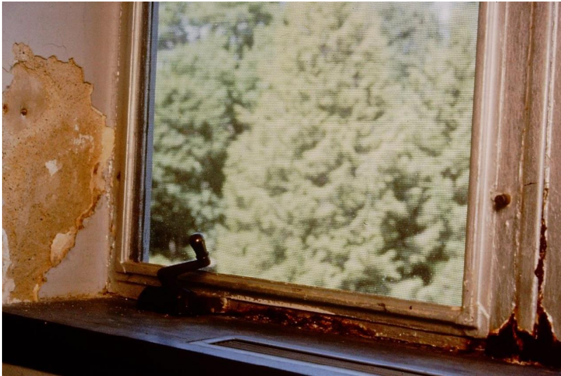
Figure 2: Interior plaster damage near window, 1985 Historic New England, Property Care Binders
