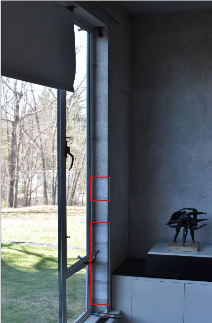
Figure 25. Location of limewash test patches (outlined in red) on window return in living room.
