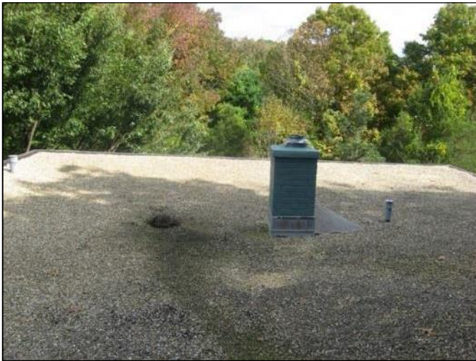
Main body of roof drain and biogrowth suggesting route of water
