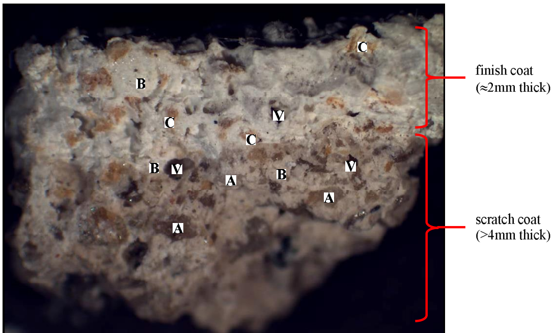
Figure 20. Cross-section of acoustic plaster with aggregate (A), binder paste (B), cellulose (C), air voids (V) and coats denoted (15X).
