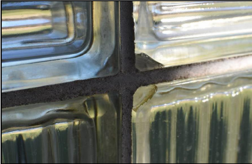
Figure 10. Typical corner spalls in glass block units.
