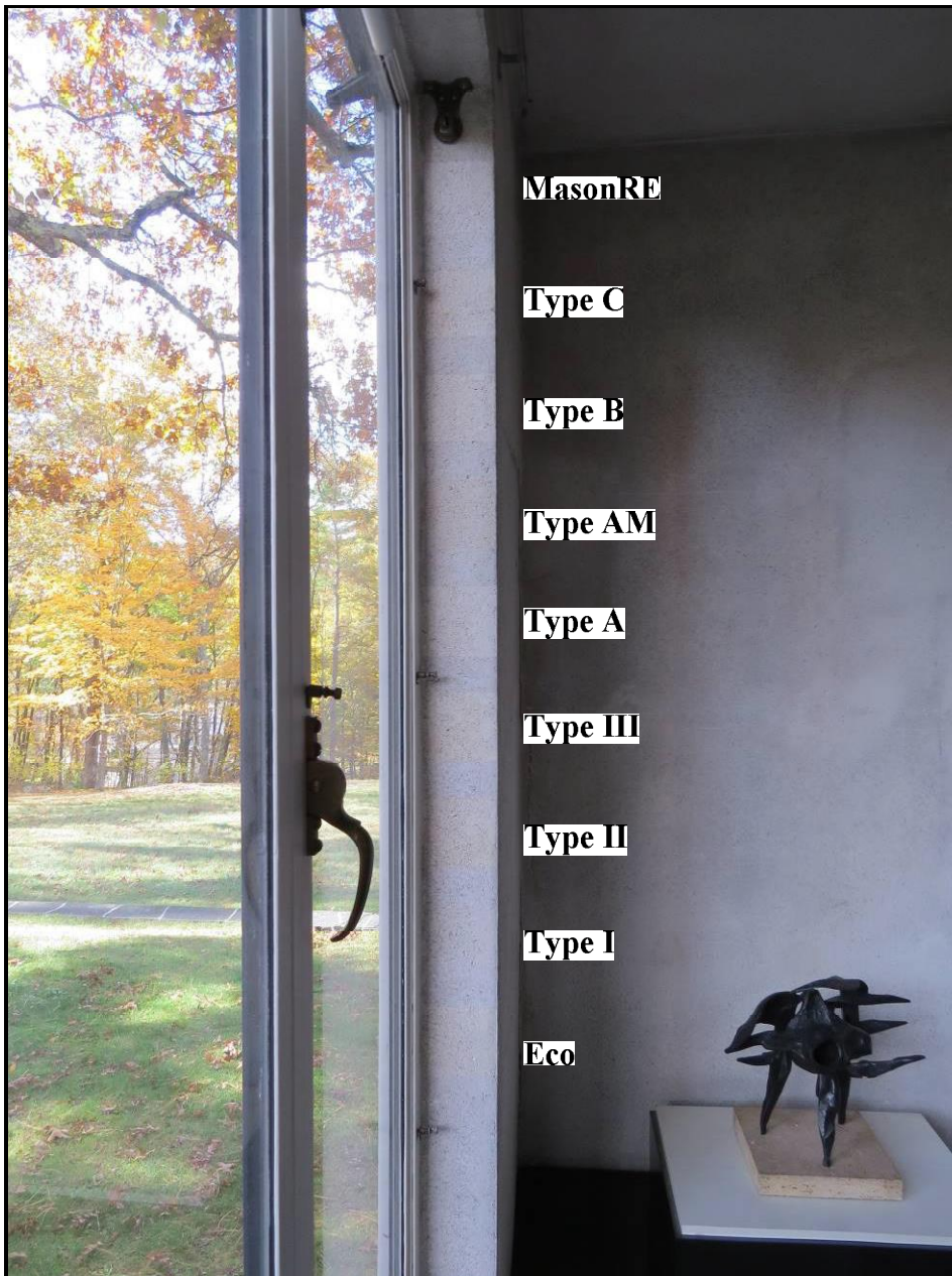
Figure 36. Poultice test area, post treatment (product names positioned next to test patch location).
