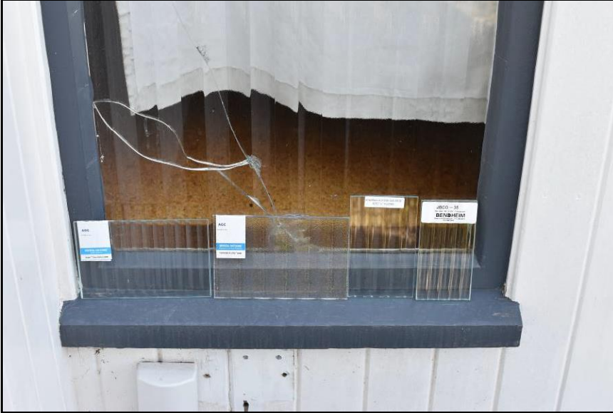
Figure 17. Samples of replacement glass compared to original Louvrex glass in Window 109 (east elevation). Samples (left to right): AGC “Flutes” Clear Pattern, AGC “Textured Flutex”, Gray Glass “1-inch Fluted”, Bendheim’s JBCO-35.
