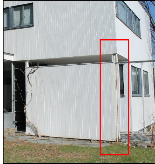
Rusted column on southeast corner
