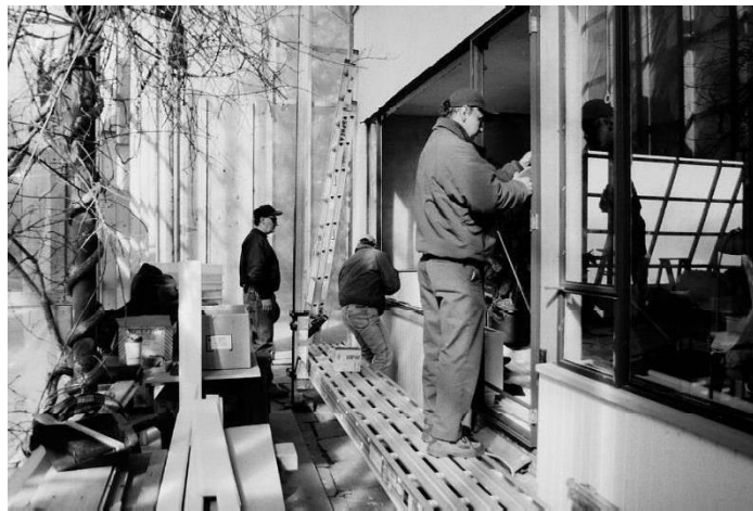
Figure 8: Window repair during the SAT grant project, 2001 Historic New England Property Care Binder, Lyman Estate
