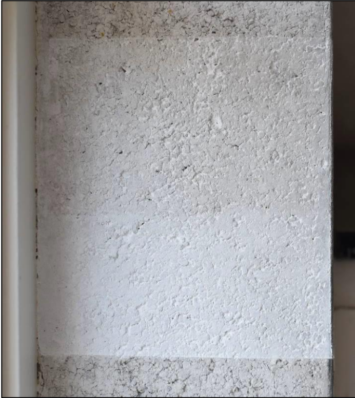
Figure 41. Brushed-on Type S limewash test patch with one (above) and two (below) coats.
