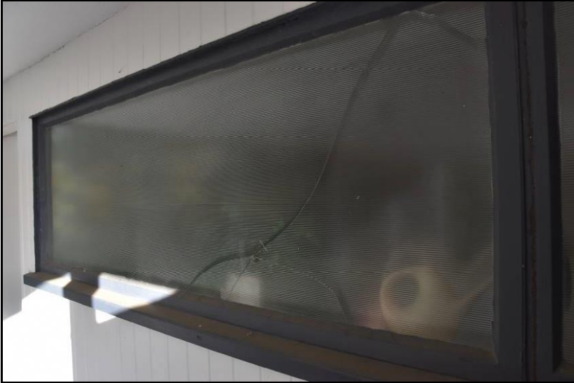
Figure 6. Stress/impact related damage in fixed-pane of Window 102.
