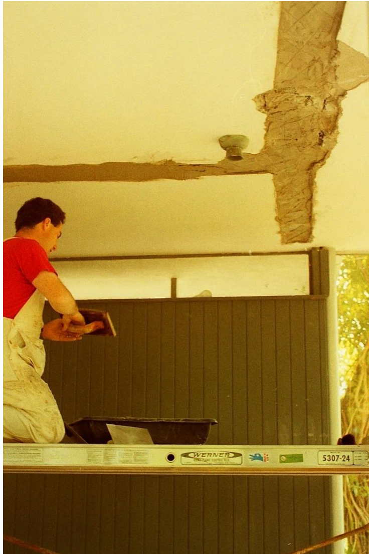
Figure 6: Porch ceiling is patched after leak repairs, 1989 Historic New England, Property Care Binders
