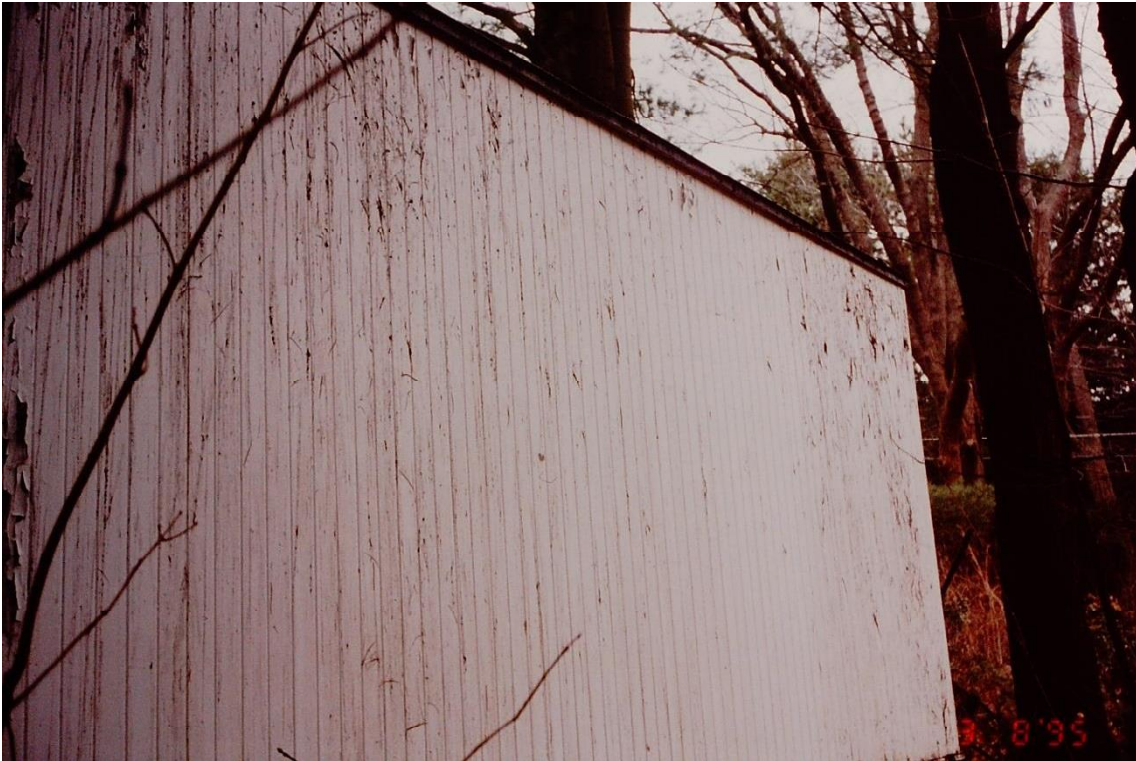
Figure 4: Damage to garage façade due to roof damage, 1995 Historic New England, Property Care Binders
