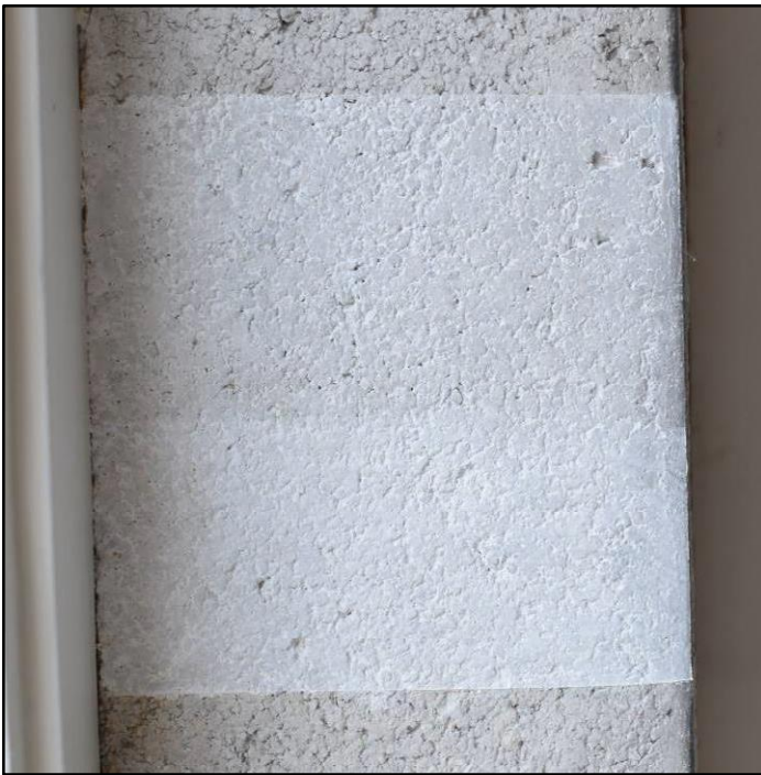
Figure 42. Brushed-on Acrylic-modified Type S limewash test patch with one (above) and two (below) coats.
