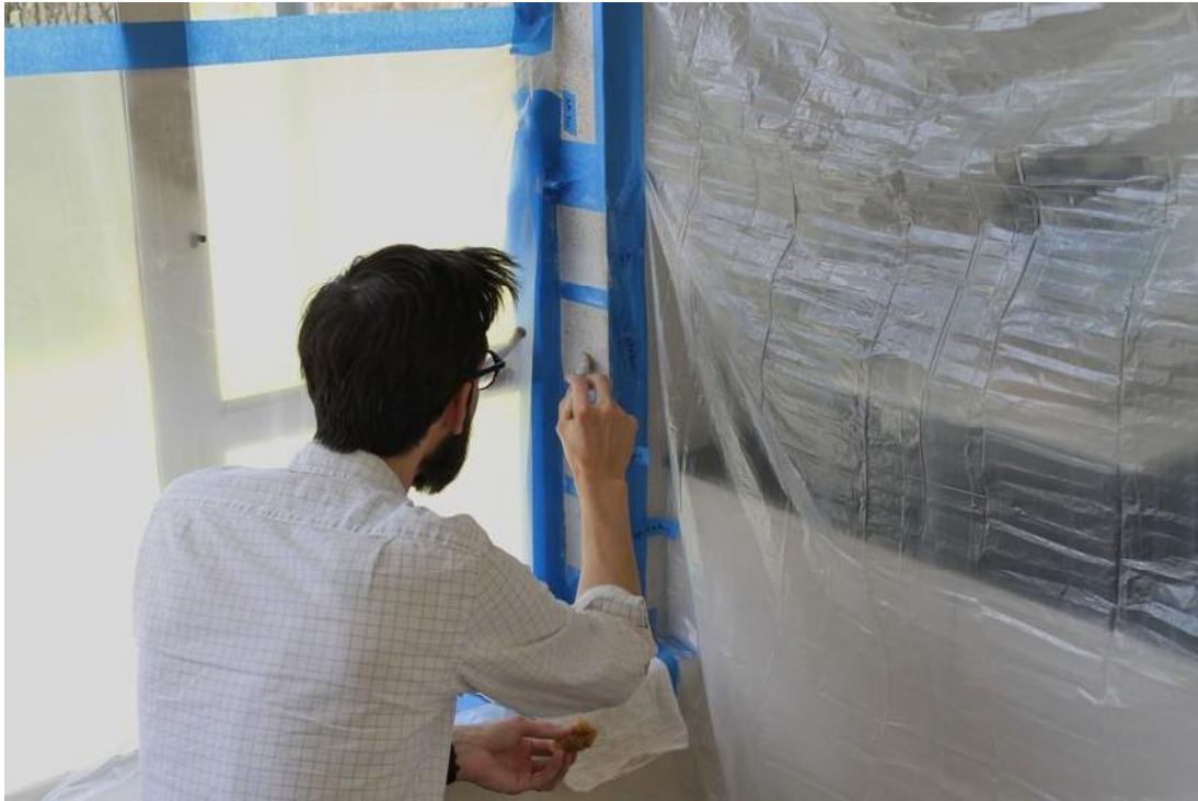
Figure 5: Ed Fitzgerald of JBC conducts testing on living room acoustical plaster, 2015 RS ID #265454
