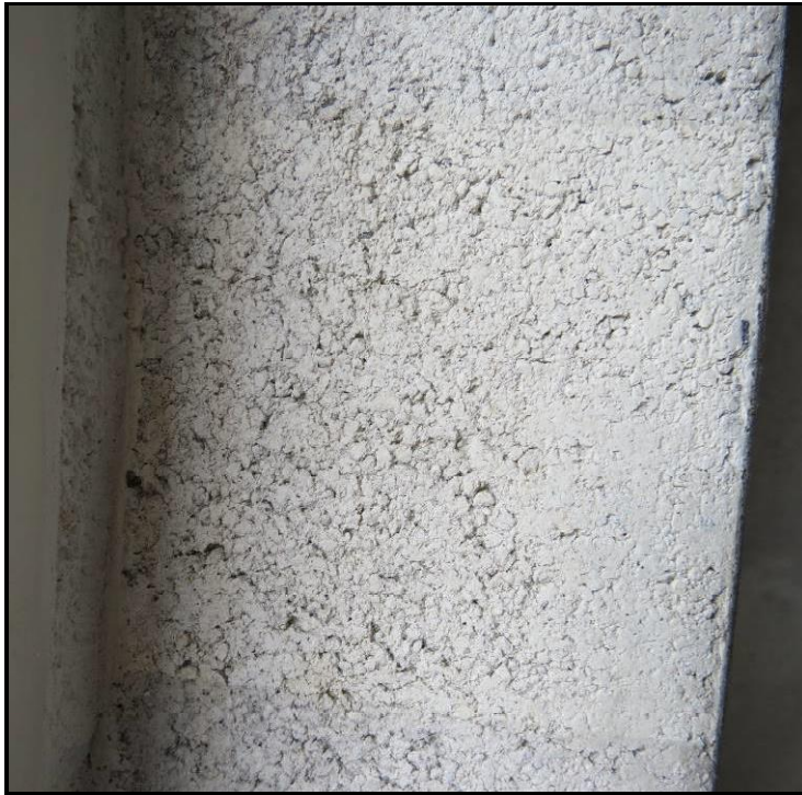
Figure 27. ABR Type A test patch, post-treatment.
