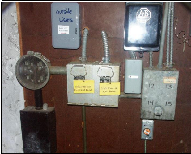
Earlier service entrance and site disconnects located at bottom of basement stairs
