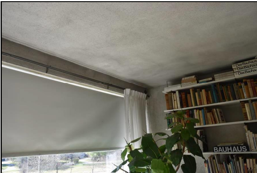
Figure 22. Typical soiling and staining observed on the plaster ceiling of the living room.
