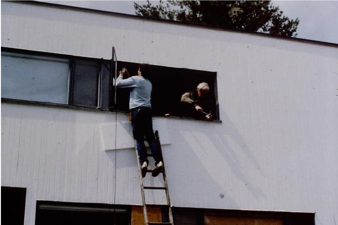
Figure 4: Repairs to east elevation windows, 1985 Historic New England Archives, Binder of Slides
