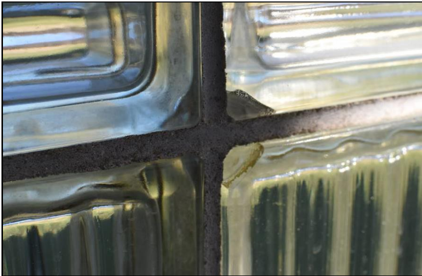
Figure 10. Typical corner spalls in glass block units.
