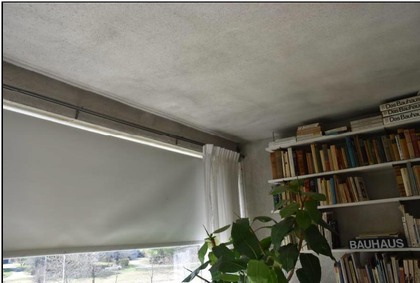
Figure 22. Typical soiling and staining observed on the plaster ceiling of the living room.
