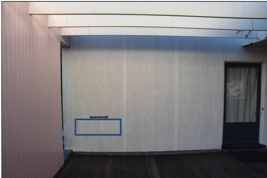
Figure 13. Cleaning test location on west elevation of the second story roof deck.
