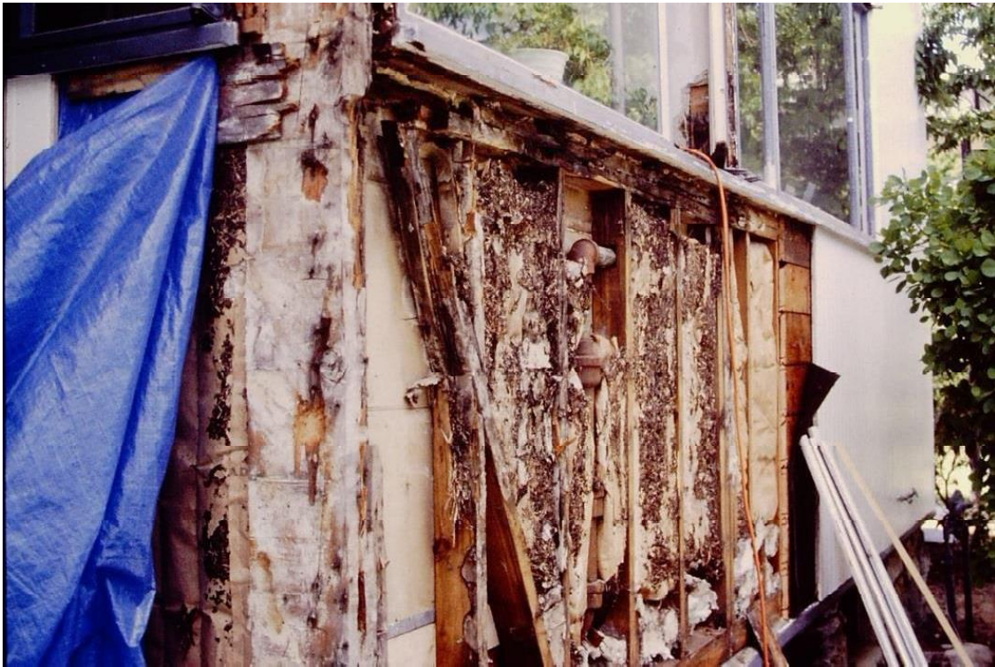
Figure 2: Deteriorating southeast corner post, 1997 Historic New England Property Care Binders
