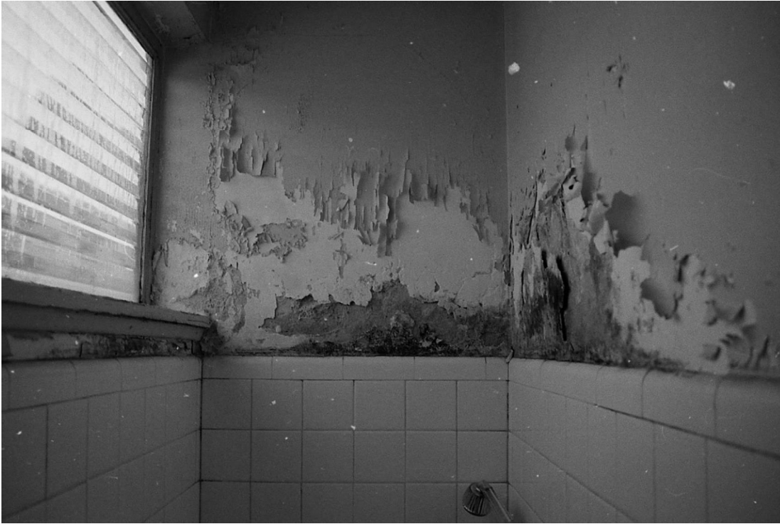
Figure 3: Damaged plaster and paint in bathroom, circa 1990s Historic New England, Property Care Binders
