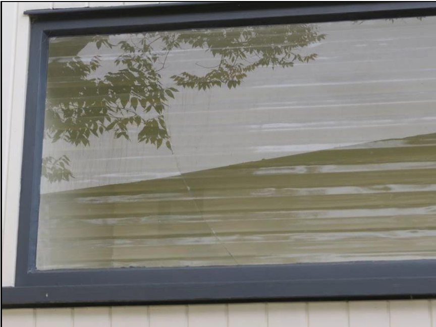
Figure 9. A single stress crack seen in Window 111.
