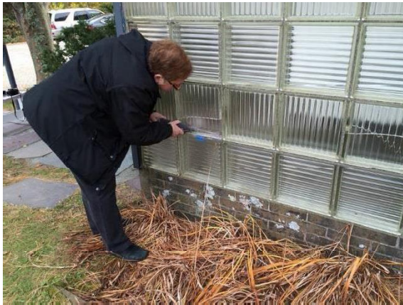
Figure 6: Mary Jablonski surveys broken glass block, 2015. RS ID #265467
