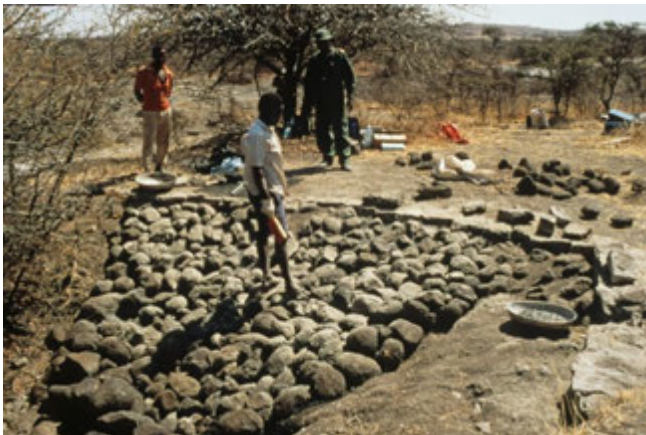
Gully stabilization near completion. Boulders were used to stabilize gully and prevent further erosion and loss of tuff.
