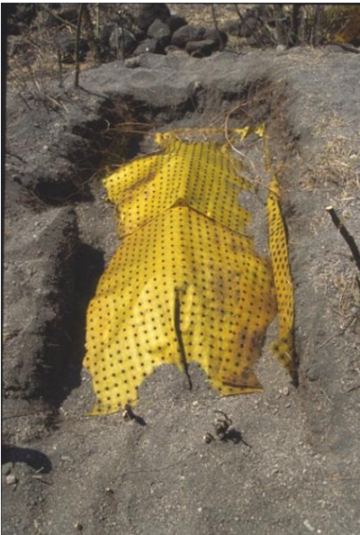
Biobarrier, a geotextile studded with herbicide nodules to inhibit root growth, was installed in the Test Site 3 trench.
