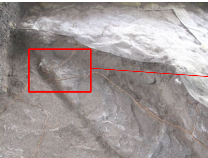
Roots penetrating tuff at edge of Fault 1. Root penetration in conjunction with excavation dislodged a piece of the tuff.
