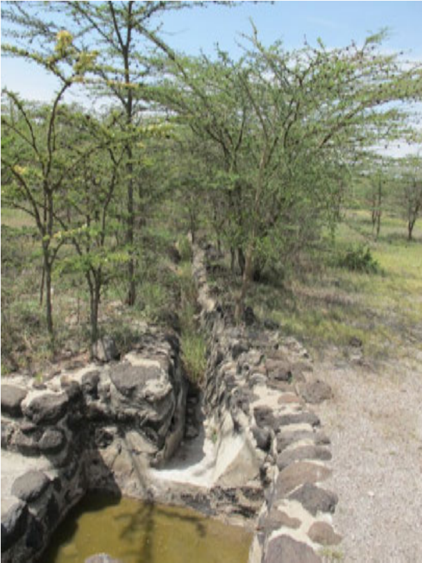
Extensive growth of acacia trees adjacent to drainage channel, which is clogged with vegetation. Catchment sump in foreground.
