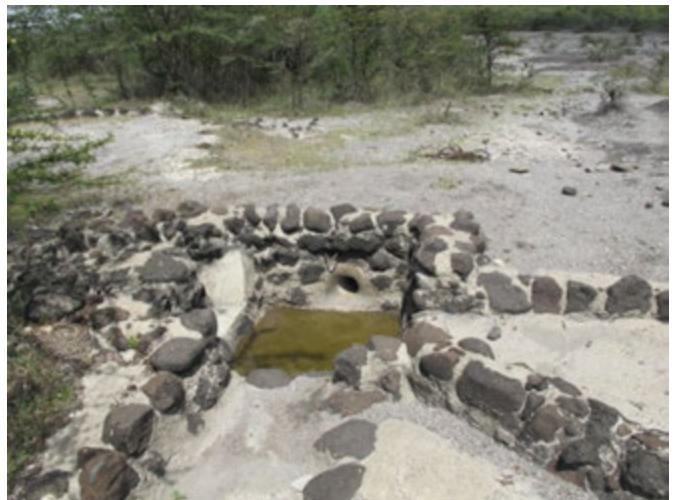
Catchment sump. Steel grill to prevent outflow pipe from clogging with vegetation is missing.
