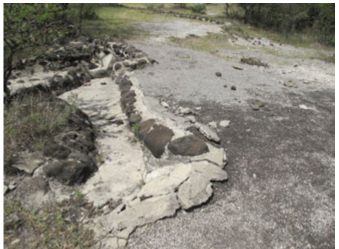
Cement inlet apron on east drainage channel is breaking up.
