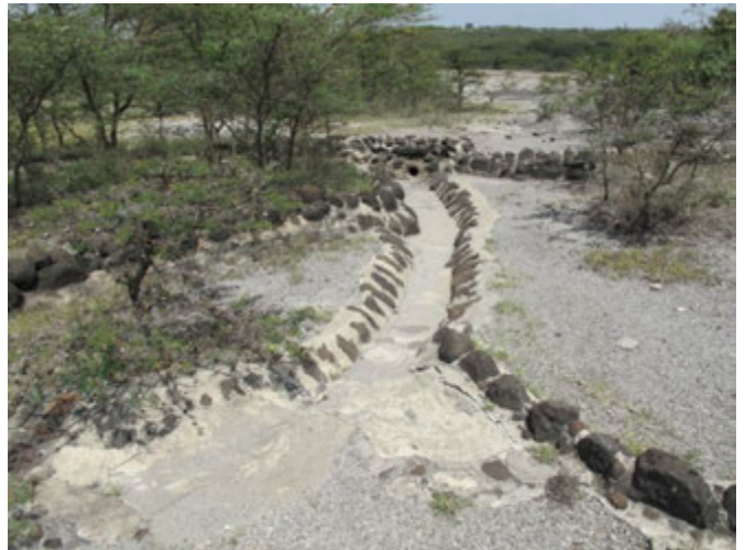
Inlet channel leading to main catchment sump; cement apron is cracking.
