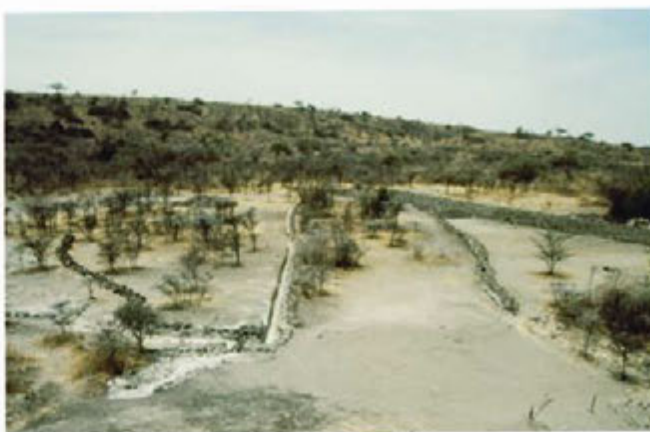
47. Site drainage control after completion: Berm 4 is in the center with Berm 2 on the left and Berm 3 on the right; looking west.
