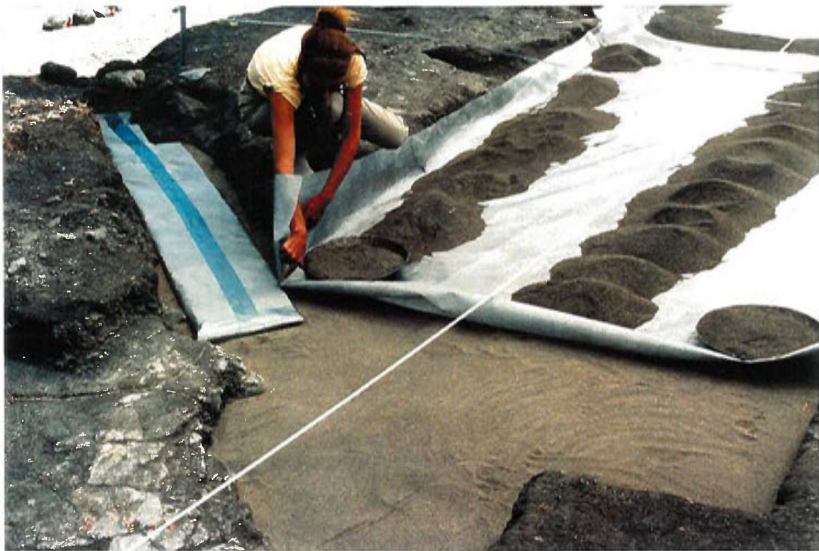
34. Early stage of the reburial showing Layer 1 in place, placement of geotextile above Layer 1 with small mounds of Layer 2 to hold it in place, and geodrain in the 1979 west trench.
