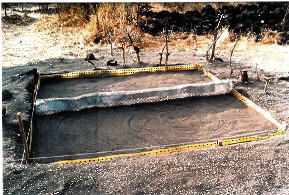
37. Test Site 3. Partial reburial of monitoring trench showing vertical placement of Biobarrier on trench walls, Layer 2 and separator barrier between north and south sections of the trench.
