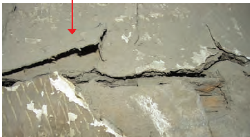
大裂缝的详图。 Detail of large crack.
