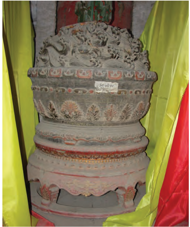
东侧珊瑚树底座。油饰地仗上有少量的脱落。 East coral tree stand. There are minor losses in the painted plaster decoration.
