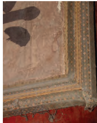
框架上的布条多处松脱。楹联表面的褐色污斑明显可见。 The fabric from the frame is coming up in places. Brown/plum colored staining is visible on the surface.
