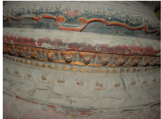
珊瑚树底座侧面图显示浮雕装饰上的裂缝和小面积脱落。 Side view of coral tree base showing showing cracks and small losses in the painted relief decoration.
