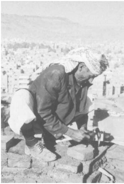
Figure 3 Ahmed al-Maswari, a master mason, perched on top of the walls of the 'Addil Mosque minaret laying bricks (1996). Photo by Trevor Marchand.
