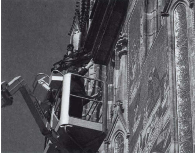
FIGURE 2 View of the mosaic's facade with conservators on a telescopic working platform. This kind of platform is necessary for monitoring and maintenance of the mosaic.
