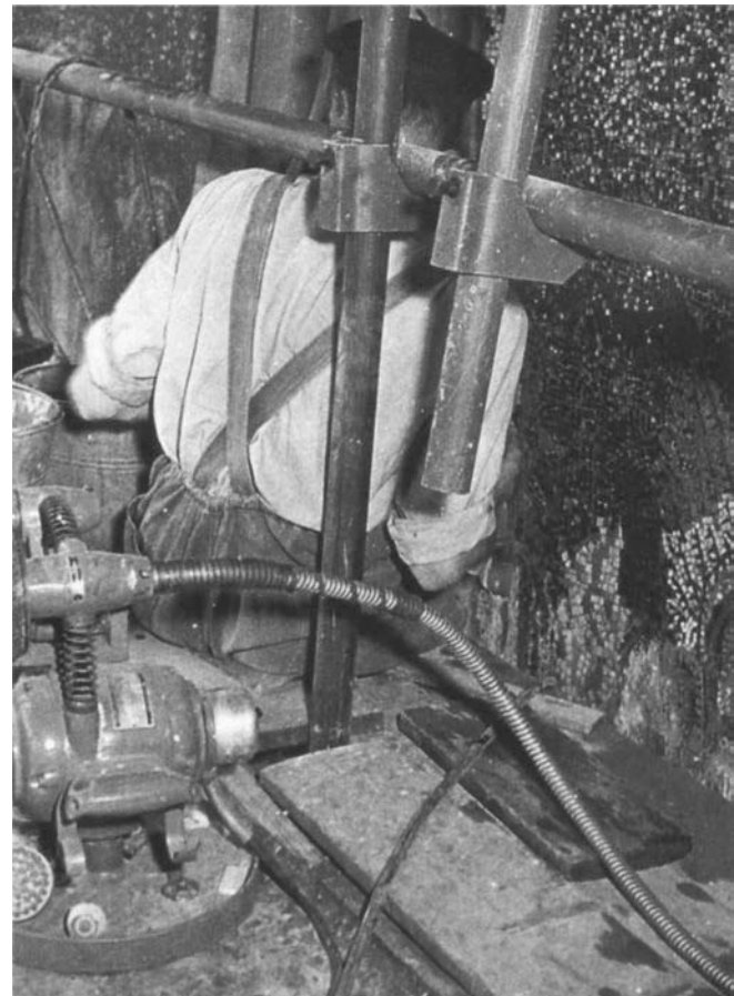
FIGURE 3 (BELOW) The corrosion was removed using wire brushes mounted on an electric motor-driven flexible shaft.
