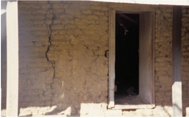
FIGURE 9 An interior wall of Las Cruces Adobe, representative of the general condition of the building. Photo: Gail Ostergren.
