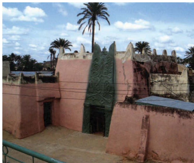
FIGURE 6 View of the Babban Gwani in 2003. Note the cracked plaster to the right of the decorated panel. Photo: Ishanlosen Odiaua.
