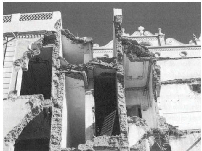
FIGURE 8 The 'Ishshah palace exemplifies the hybrid of imported colonial styles executed in the local construction technology of mud-brick and lime plaster. A large section of the west elevation collapsed in 2000 and was reconstructed in 2003 through the efforts of the Tarimi Mansions Preservation Project.
