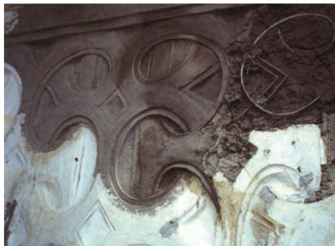
FIGURE 6 White wall during restoration, showing the palm stick reinforcements inserted in the clay (Edwenase shrine). Photo: Sébastien Moriset, CRATerre-EAG.
