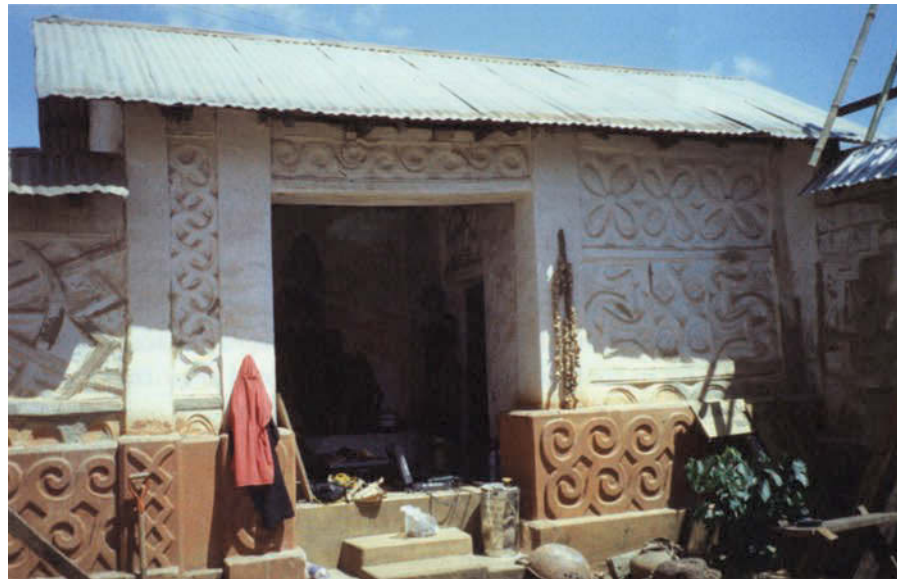
FIGURE 7 Besease shrine before the replacement of the roof with a replica of the steep traditional roof covered with raffia thatch. Photo: Thierry Joffroy, CRATerre-EAG.
