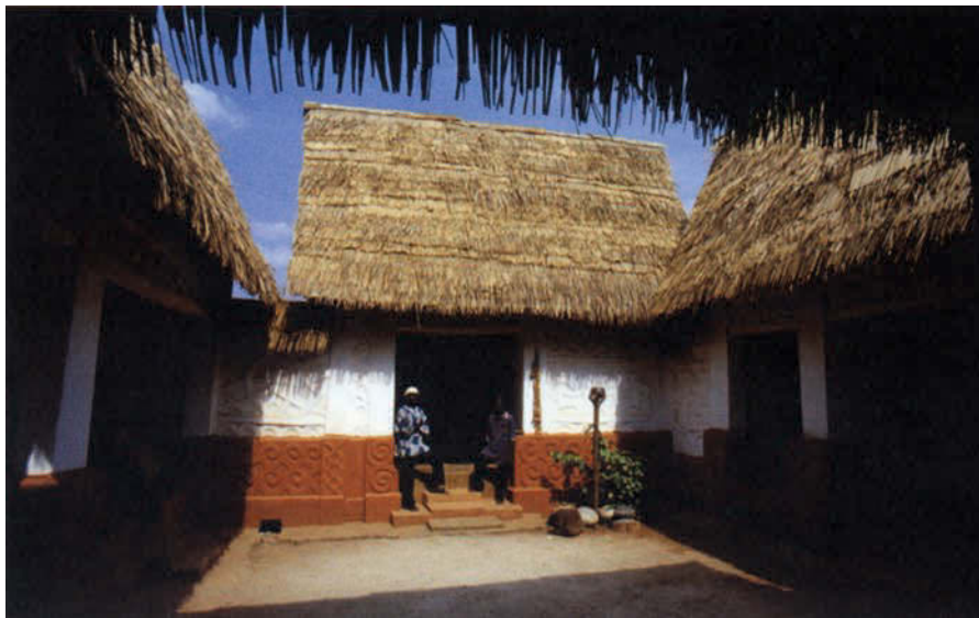
FIGURE 9 Besease shrine after the replacement of the corrugated iron sheet roof with a steep traditional roof, made of wood, bamboo, and raffia thatch. Photo: Thierry Joffroy, CRATerre-EAG.
