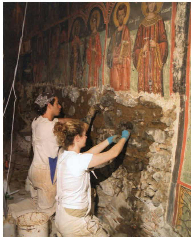
FIGURE 6 Repointing of the stone plinth using the tested repair mortar. Photo courtesy of the Courtauld Institute of Art, Conservation of Wall Painting Department, 2002.
