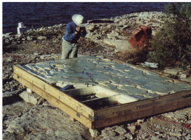
FIGURE 8 The frame and wall painting with its temporary backing, designed to sandwich the wall painting while in transit (February 2003). The timber mold constructed around the edges of the plaster can be seen. A foil barrier was created on the plaster, and several pours of polyurethane foam cast into the back. The plywood lid, which had been used to contain the foam during casting, was then screwed on to complete the packing process. Courtesy of the Egypt Exploration Society.
