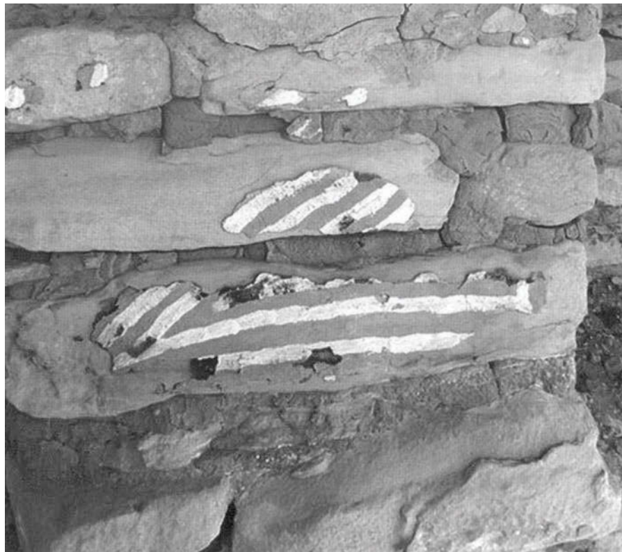
FIGURE 1 The advanced deterioration of a kiva pilaster in Kodak House is attributed to its exposure to an outside environment. The surface finishes on this interior architectural feature were exposed to weathering after the roof of this kiva collapsed. Courtesy of ASCP Digital Archives, Mesa Verde National Park. Photo: Laurel Casjens.
