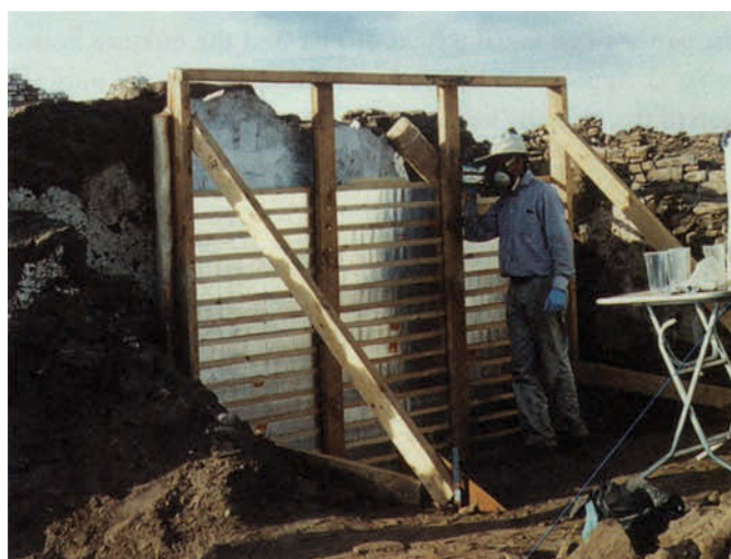
FIGURE 5 The rectangular timber frame in place, supported by an A-frame at each end (February 2003). The process of building up the shuttering and pouring in the polyurethane foam is two-thirds complete. Courtesy of the Egypt Exploration Society.
