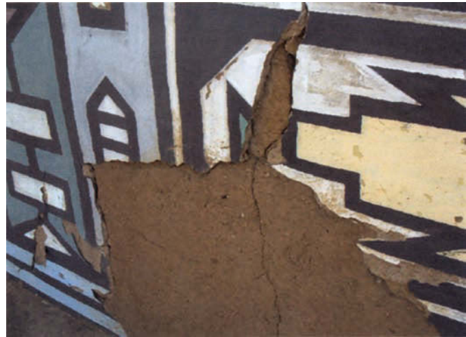
FIGURE 7 Damage resulting from the use of cement additives. Here typical delamination and structural failures can be seen where the cement plaster layer has become detached from the original mud plasterwork of a Klipgat home. Photo: K. A. Bakker, 2004.
