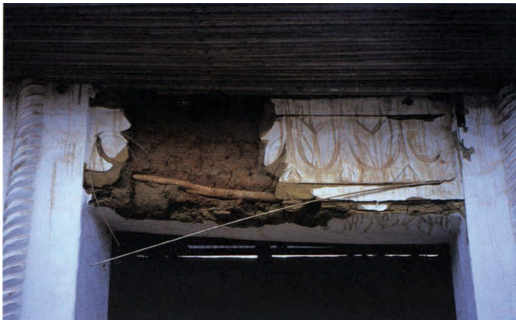
FIGURE 3 Decorated beam, damaged after the displacement of a roofing sheet during a rainstorm (Patakro shrine). Photo: Sébastien Moriset, CRATerre-EAG.
