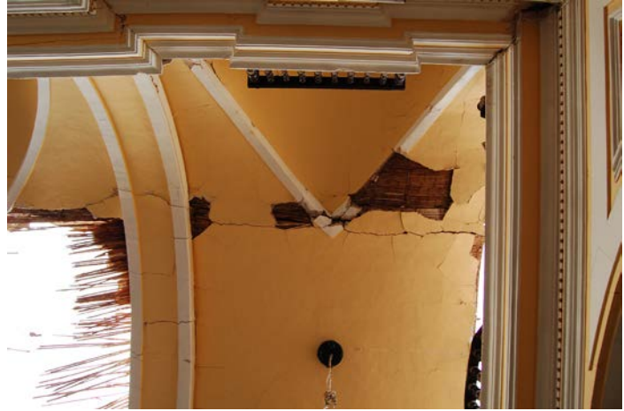
FIGURE 4.14 View of crack where partial collapse of the vault occurred at the Cathedral of Ica, as seen in October 2007.
