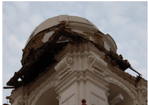
FIGURE 4.32 Displacement of upper dome due to failure of connections with tower pillars, Church, Hacienda San José, Cañete, as seen in October 2007.
