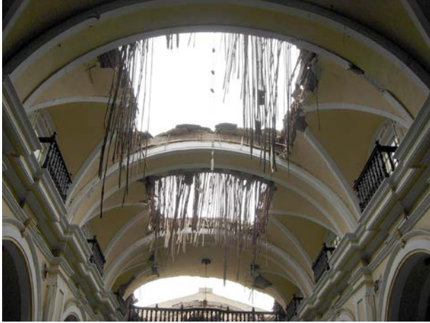
FIGURE 4.13 Detail of vault failure in the main nave of Cathedral of Ica following the Pisco earthquake, as seen in October 2007.
