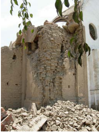
FIGURE 4.37 Detail showing the mixture of building materials used at the Church of Coayllo, as photographed in October 2007.
