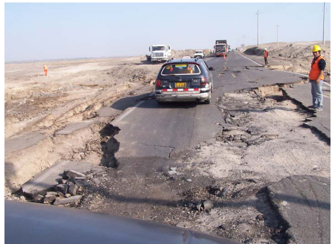
FIGURE 2.19 Landslide effects at the Pan-American Highway.
