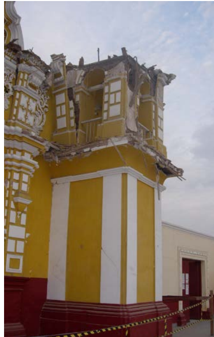
FIGURE 4.7 Detail showing total collapse of church tower dome at the Church of El Carmen in Chincha, as it appeared in October 2007.
