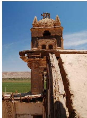
FIGURE 4.31 Separation of main façade from vault at the Church of Hacienda San José de Nazca, as seen in October 2007.
