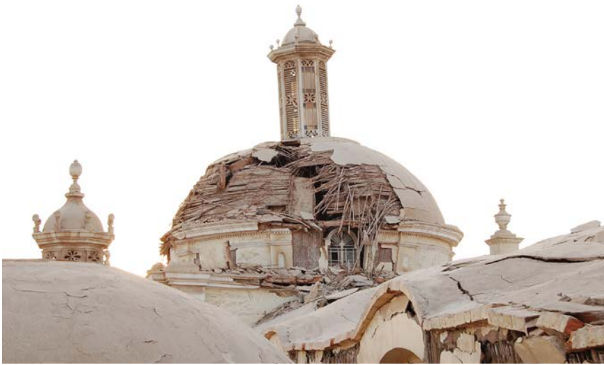
FIGURE 4.28 Plaster detachment on the dome of the Cathedral of Ica, as seen in October 2007.
