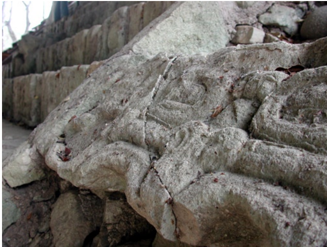
Figure 88 A crack in a large horizontal stone (6S-107) of the south balustrade, near step 37.
