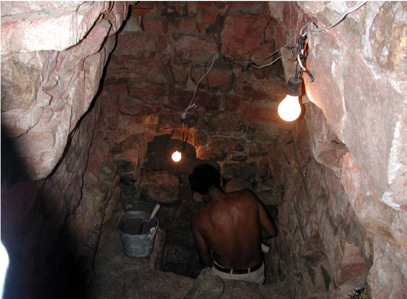
Figure 90 View of a tunnel in the Margarita Tomb, showing work in progress.
