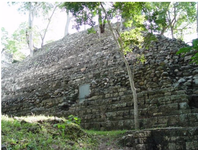
Figure 92 A small tree growing on the north end of the east face of Structure 26; it could easily be removed before it grows to a damaging size.
