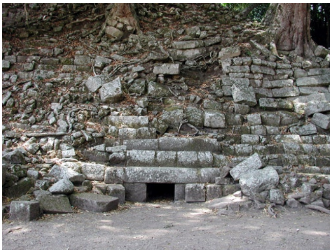
Figure 93 An ancient drain outlet in the southwest corner of the Court of the Hieroglyphic Stairway.
