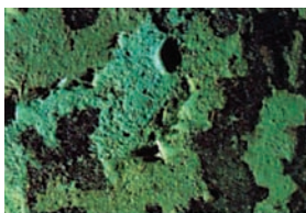
FIGURE 8. Area of the monument showing both older and more recent coatings with sections of the latter peeling away from the older corrosion patina.
