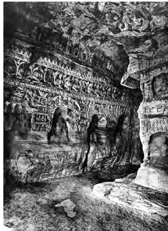
FIGURE 1 Weathering of the lower part of the west wall of cave 1 due to groundwater.
