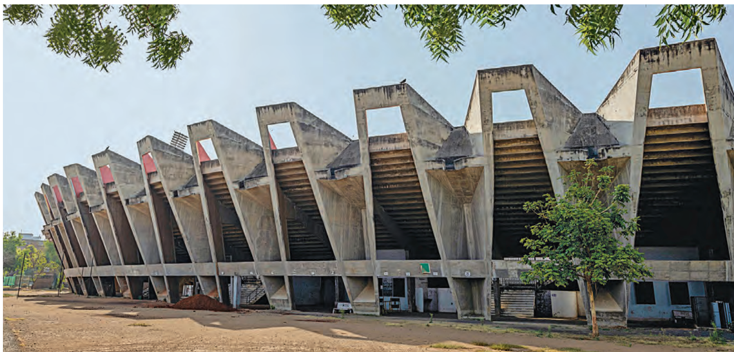
Sardar Vallabhbhai Patel Stadium in Ahmedabad, India. This cricket stadium—designed by architect Charles Correa and engineer Mahendra Raj and completed in 1960—was included on the 2020 WMF Watch list, which was followed by a multidisciplinary project, with Getty support, to prepare a conservation and management plan for the site. Photo: Sanat Jhaveri & Co. Image courtesy of the World Monuments Fund.
