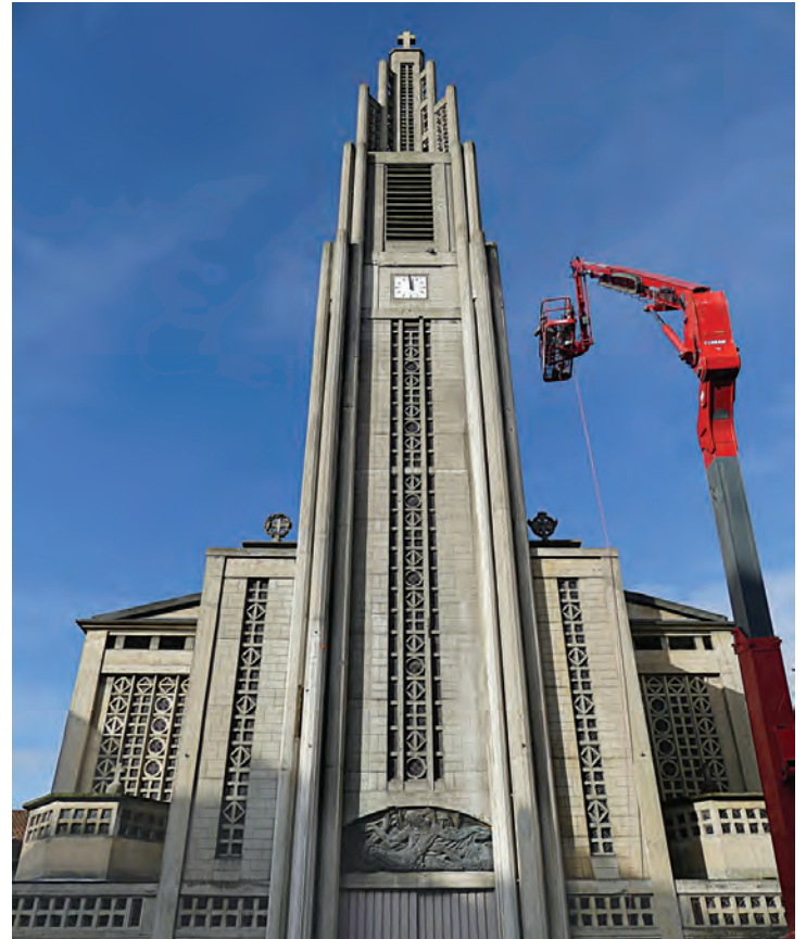
Notre-Dame du Raincy , designed by Auguste and Gustave Perret and completed in 1923. This masterwork of early reinforced-concrete construction was one of France's first concrete churches and is now a research project site of PEPS, a collaboration with Historic England and the Laboratoire de Recherche des Monuments Historiques (France). Here, the team is undertaking investigations of earlier concrete patch repairs to the bell tower. Photo: @LRMH.
