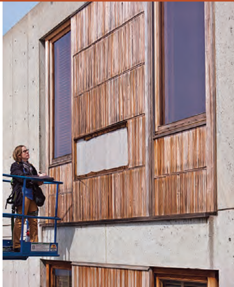
Sara Lardinois of the GCI assessing a teak wall at the Salk Institute in 2014. The GCI partnered with Salk to address the long-term care of the building's teak window wall assemblies, a major element of the architectural ensemble. Photo: Jeffrey Levin, GCI.
