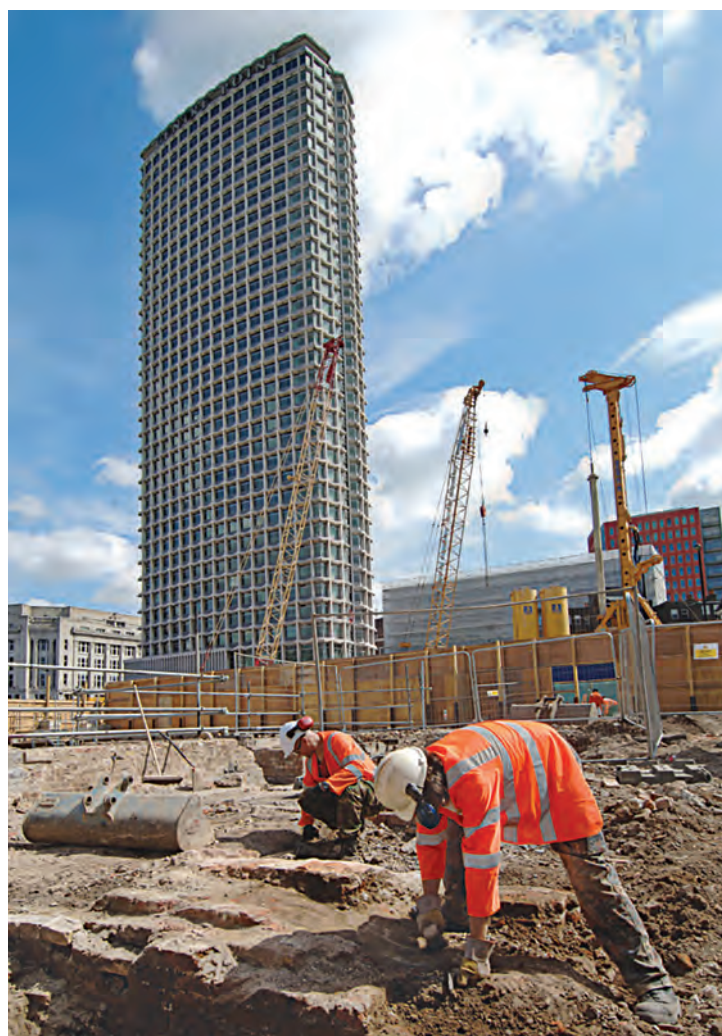
Excavation related to the redevelopment of parts of Tottenham Court Road Underground Station in London's West End by Crossrail Ltd. The vast majority of UK archaeological work undertaken each year is development-led or commercial archaeology, and the ADS has prioritized making information about these projects broadly available. Photo: © Museum of London Archaeology CC-BY 4.0.
