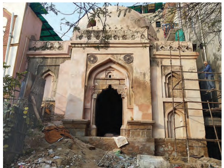
Before and during conservation of a 15th-century Lodhi period tomb in the urban village of Lado Sarai in South Delhi. The area around the tomb is now dense, unplanned development. Conservation work started in 2019, but progress has been delayed because of the difficult site condition and the restrictions imposed to contain the COVID-19 pandemic. Photo: Courtesy of the INTACH Delhi Chapter.
