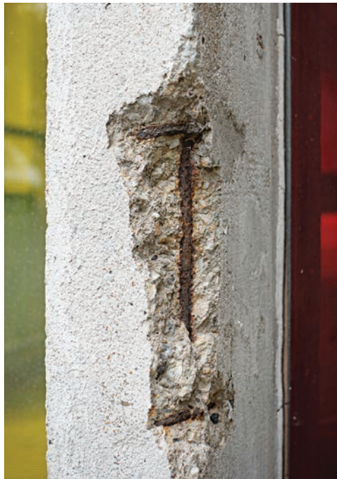
Concrete spall due to corrosion in the steel reinforcement. Photo: Ana Paula Arato Gonçalves, GCI.
