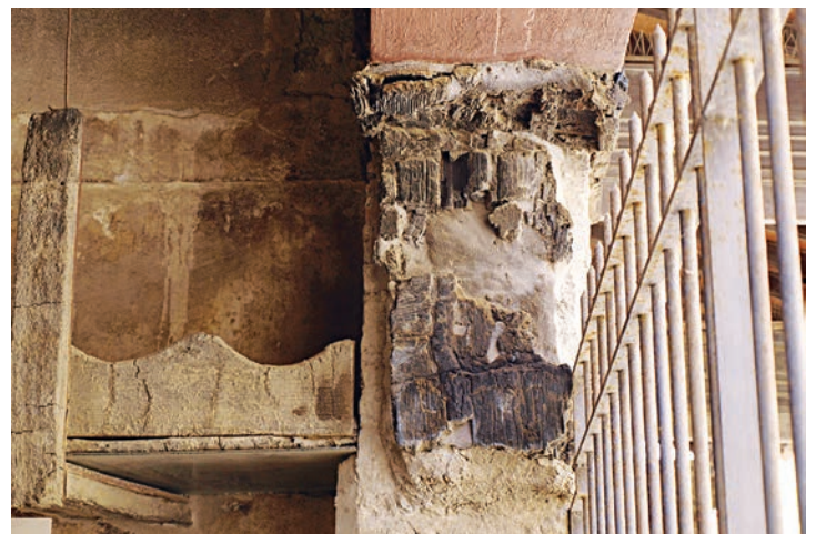
A lintel and post in reinforced concrete covered with Roman carbonized wood. The site is one of the shops on the Decumanus Maximus (Bottega del Plumbarius). Photo: Herculaneum Conservation Project.
