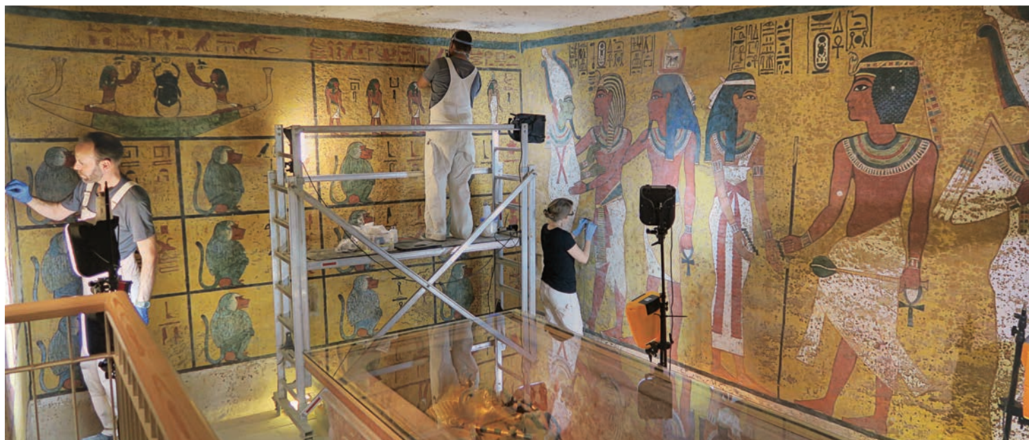
Wall painting conservation work being conducted in the burial chamber of the tomb in spring 2016. Photo: Neville Agnew, GCI.
