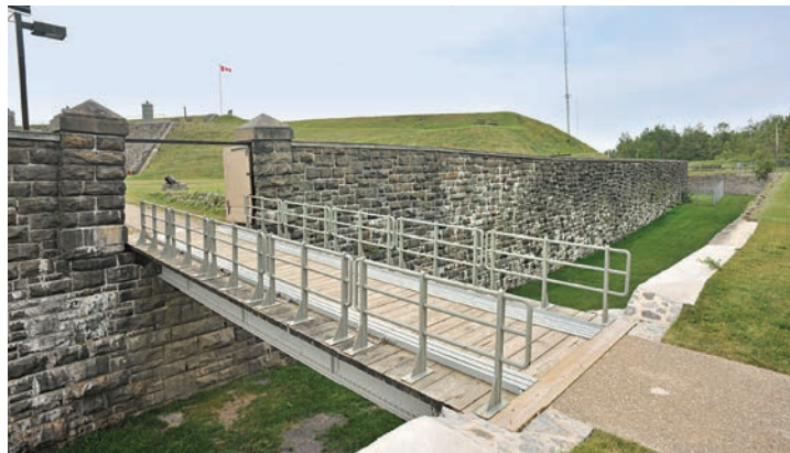
Above: A fortification wall at Lévis Forts National Historic Site of Canada, Fort No. 1. Top: A single photogrammetric model shows that the wall is out of plane by 0.7 meters (3 feet). Photo/Image: HCS, Technical Services, Public Services and Procurement Canada.
