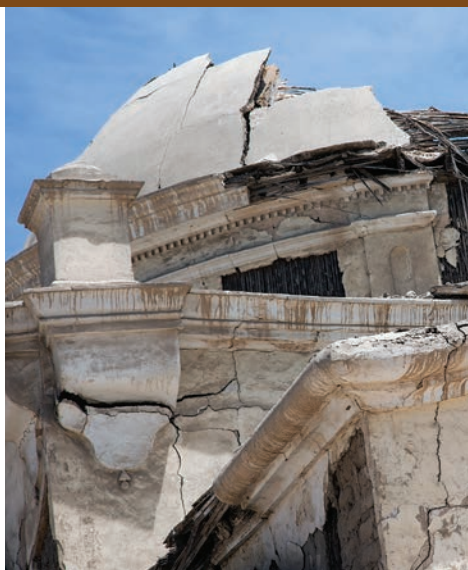
A detail of exterior earthquake damage to Ica Cathedral in Peru. Photo: Scott S. Warren, for the GCI.
