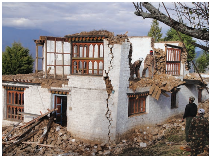
A traditional house in East Bhutan, heavily damaged by earthquake in 2009. Photo: Rohit Jigyasu.
