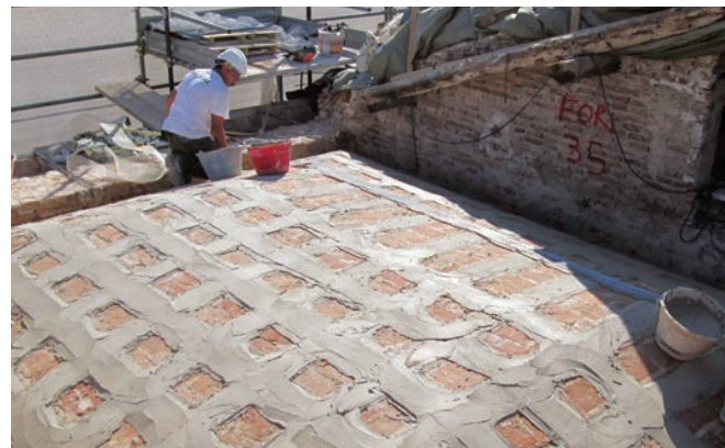
Steel-reinforced grouts (SRG) being applied as reinforcement to a vault in L'Aquila, Italy. Photo: Gianmarco de Felice.
