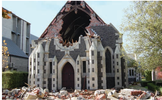
The 1910 Rose Historic Chapel in Christchurch, New Zealand, damaged during the Christchurch earthquake in 2011. Photo: João Leite. Courtesy of Paulo B. Lourenço.
