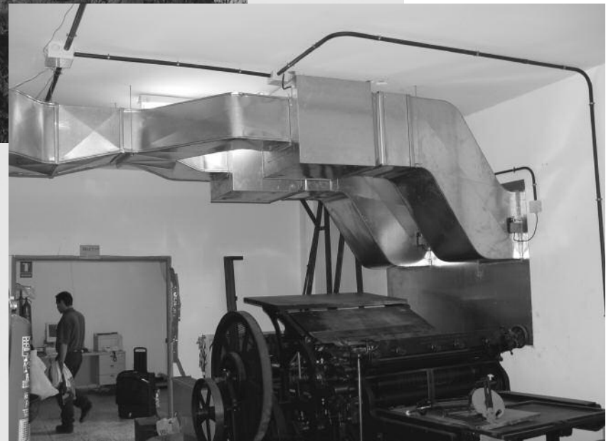
Above left: The Valle de Guerra museum storage facility in Tenerife. Above: A view of the facility's ventilation system. Ducting of the ventilation system was necessary as two walls of the storage area are devoid of windows. Here, two supply ventilators are connected to one ventilation duct to create high-volume airflow into the storage space. Photos: Shin Maekawa.
