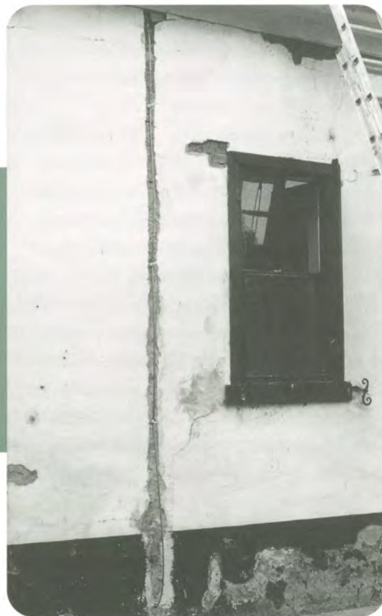
Left: A vertical steel cable recessed into an exterior wall. The cable will be prestressed, then covered with adobe mortar.
