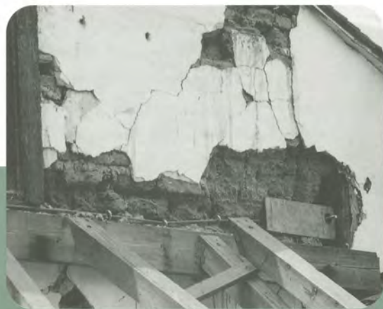
Above: A detail of the east gable during repair and seismic retrofitting. Visible is a horizontal steel cable with cable ties, and a stress distributing end plate. Photo: William S. Ginell.
