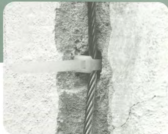
Below: A detail of a steel cable and nylon tie. Photos: William S. Ginell.
