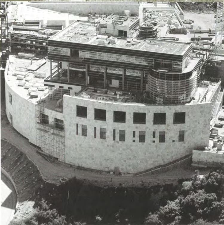
Top: The Getty Center under construction in June 1995. Bottom: The building at the Center that will house the Getty Conservation Institute. Photos: Warren Aerial Photography.
