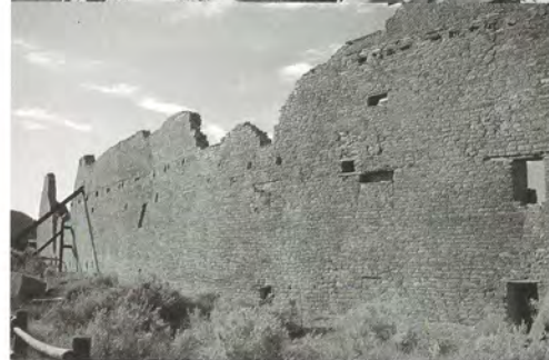
Top: At the Anasazi ruins in Chaco Canyon, New Mexico, Mike Taylor of the U.S. National Park Service and Neville Agnew of the GCI examine geosynthetic material installed to protect the stone walls from water damage. Bottom: The north wall of Pueblo Bonito at Chaco Canyon. Photos: Guillermo Aldana.
